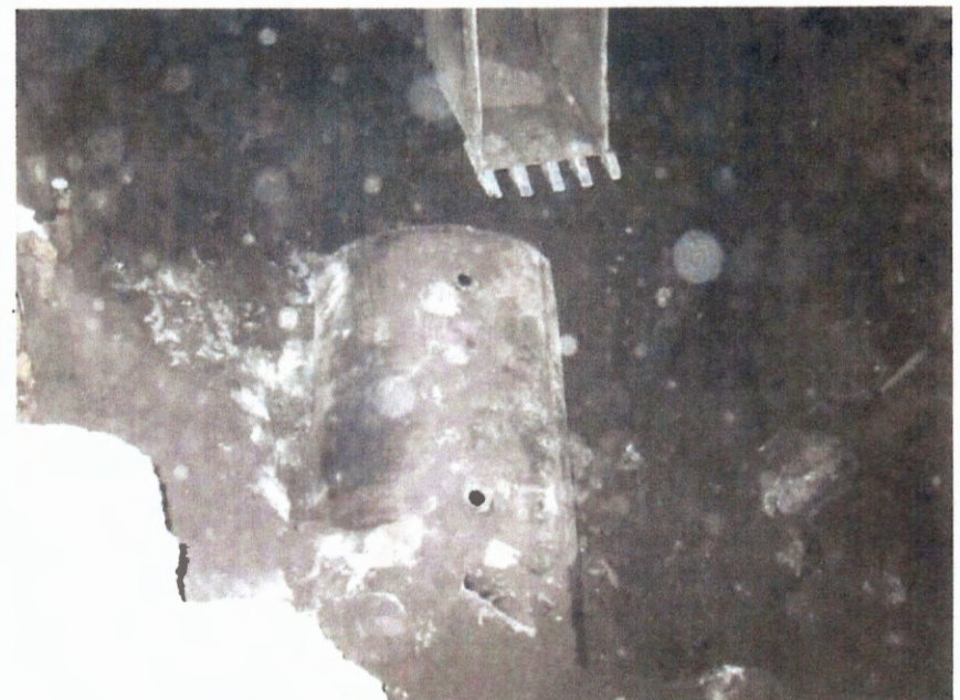
SOUTHERN TANK EXPOSED
