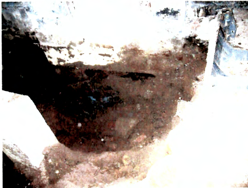
EXCAVATION SHOWING LEAK SOURCE
