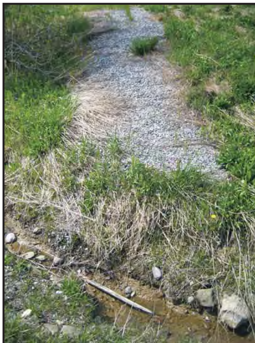
Photo 2: Gravel drainage area at east end of north permeable reactive wall.
