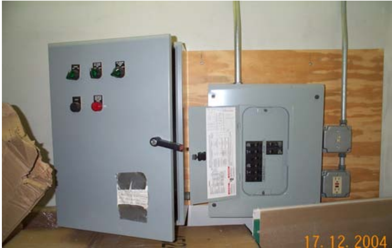
Outside of control box for the AS/SVE system (LA Furniture).
