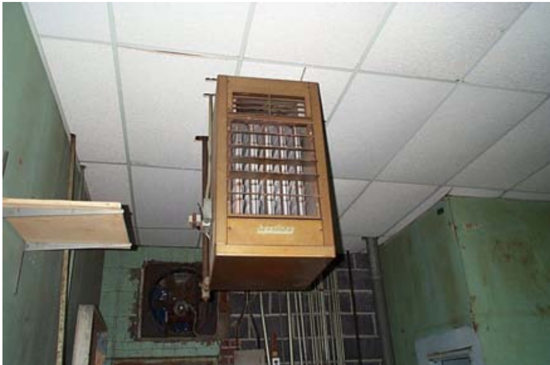
HVAC intake located in LA Furniture
