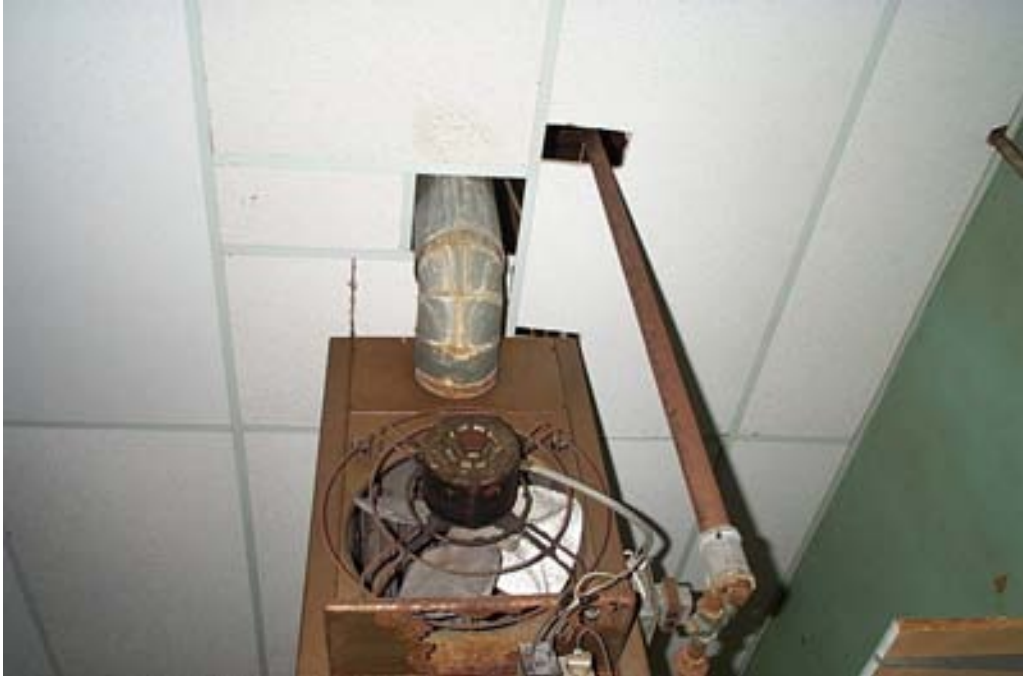
Photograph of the other side of the HVAC system
