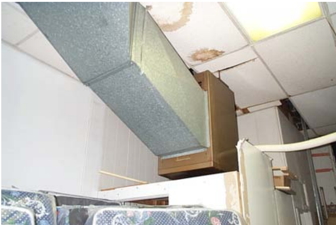
Ceiling vent located in LA Furniture outside the room containing SVE/AS system
