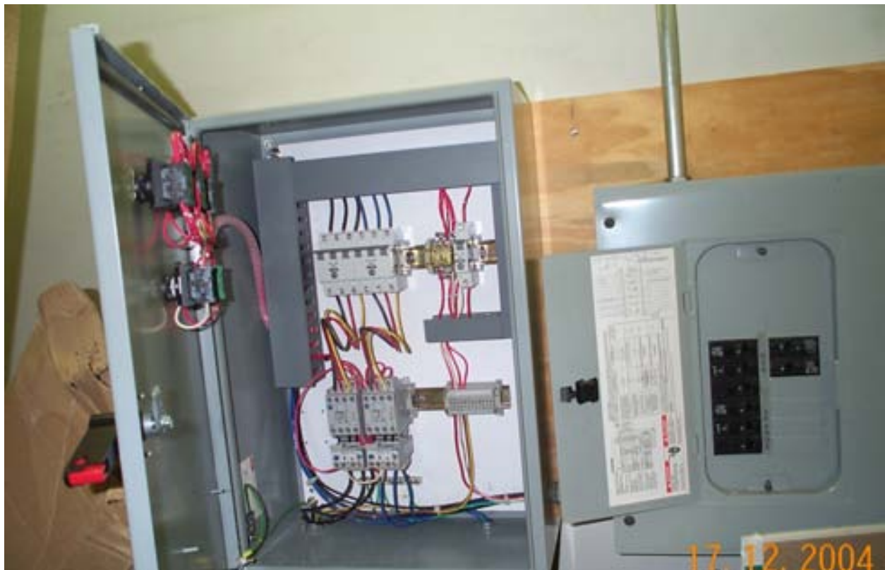
Inside of control box for the AS/SVE system (LA Furniture).
