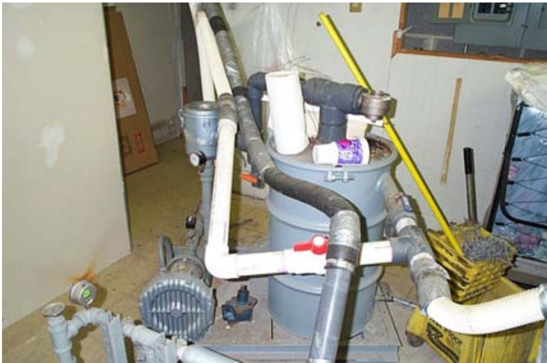
View of SVE/AS system located in LA Furniture
