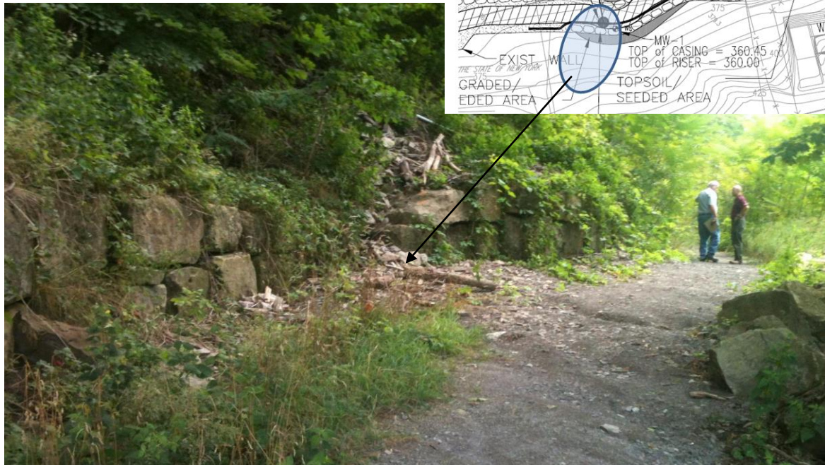
Overview showing the block wall to the north and south of the landslide area near SW-2. MW-1 is located a few yards east of SW-2 and has the same type of stone block wall protecting it. Movement of the slope is slowly pushing the adjacent stone over the monitoring well.
