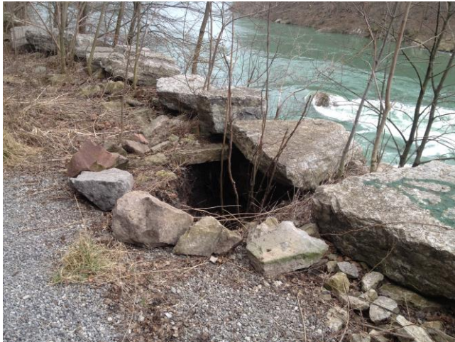
SINK HOLE BY LOWER RETAINING WALL; UPPER RETAINING WALL TO THE LEFT
