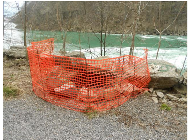
TEMPORARY SAFETY FENCE AT SINK HOLE
