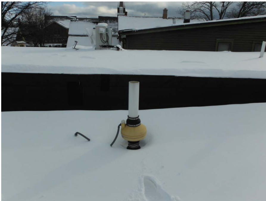
Photograph 2 – Southern SSV Mitigation Roof Fan
