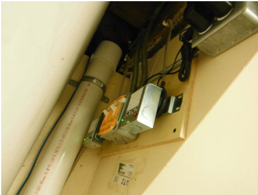
Photograph 4 – SSV Mitigation System Controls and Monitoring Equipment
