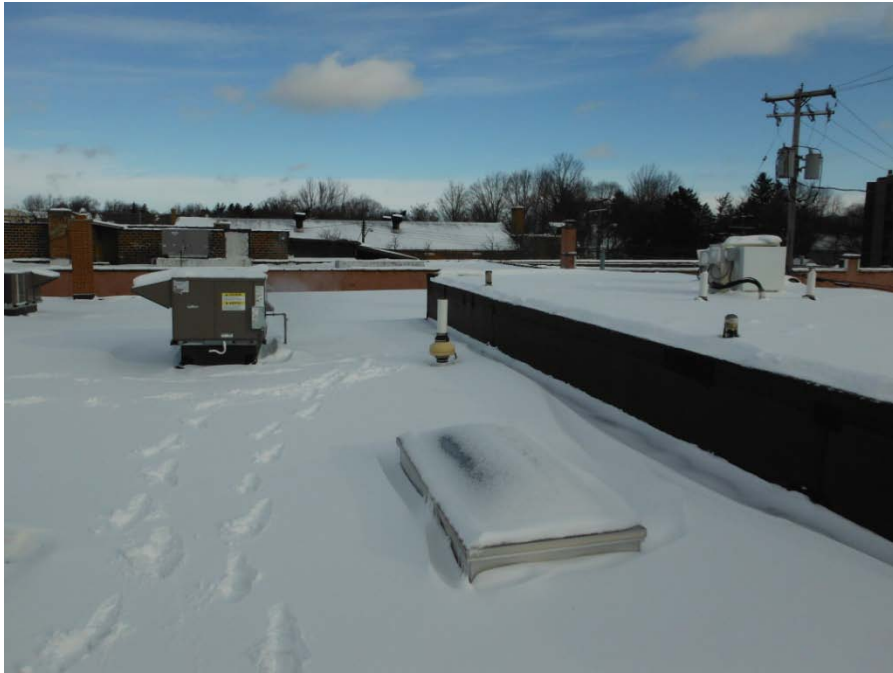
Photograph 1 – Northern SSV Mitigation Roof Fan
