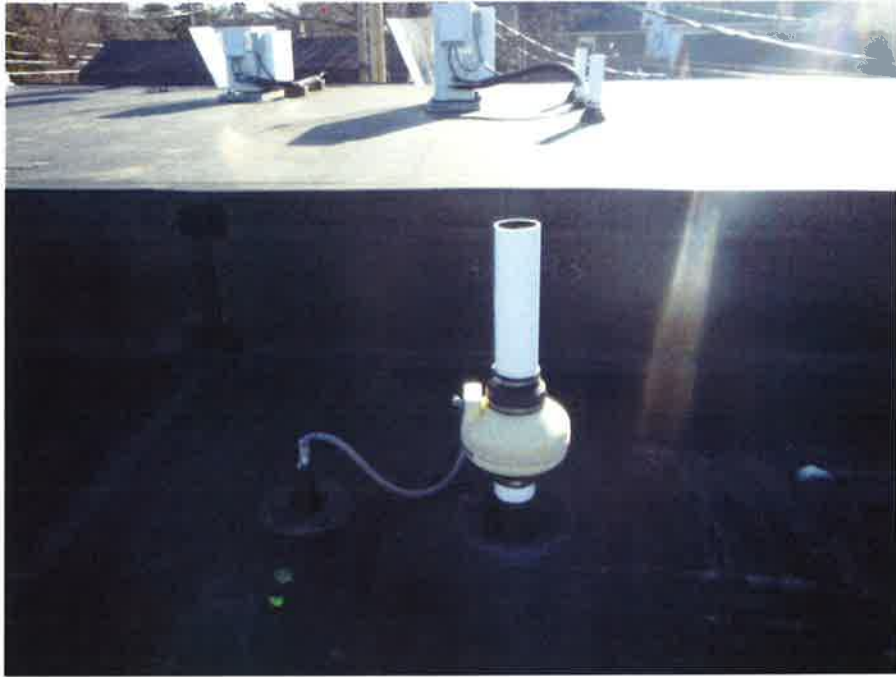
Photograph 1 – Northern SSV Mitigation Roof Fan
