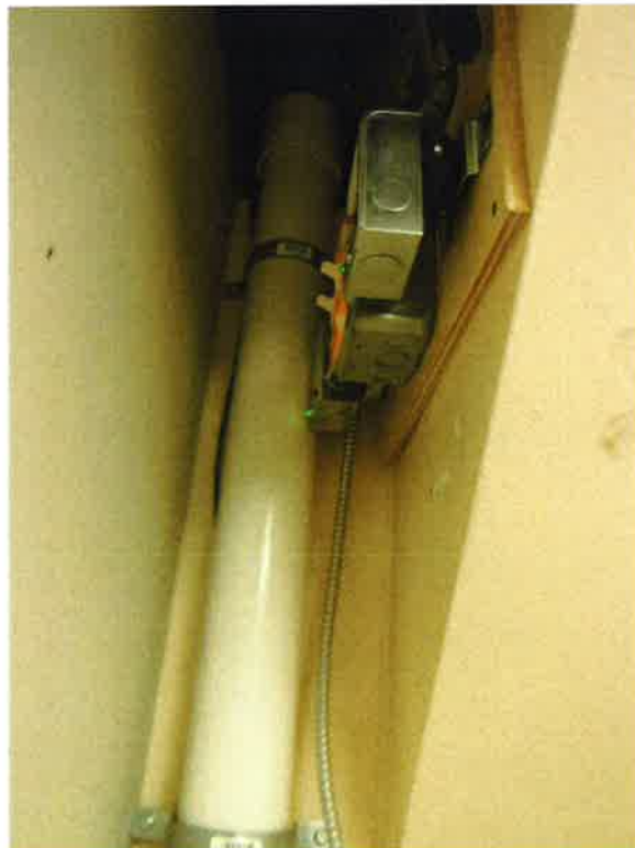
Photograph 4 – SSV Mitigation System Controls and Monitoring Equipment
