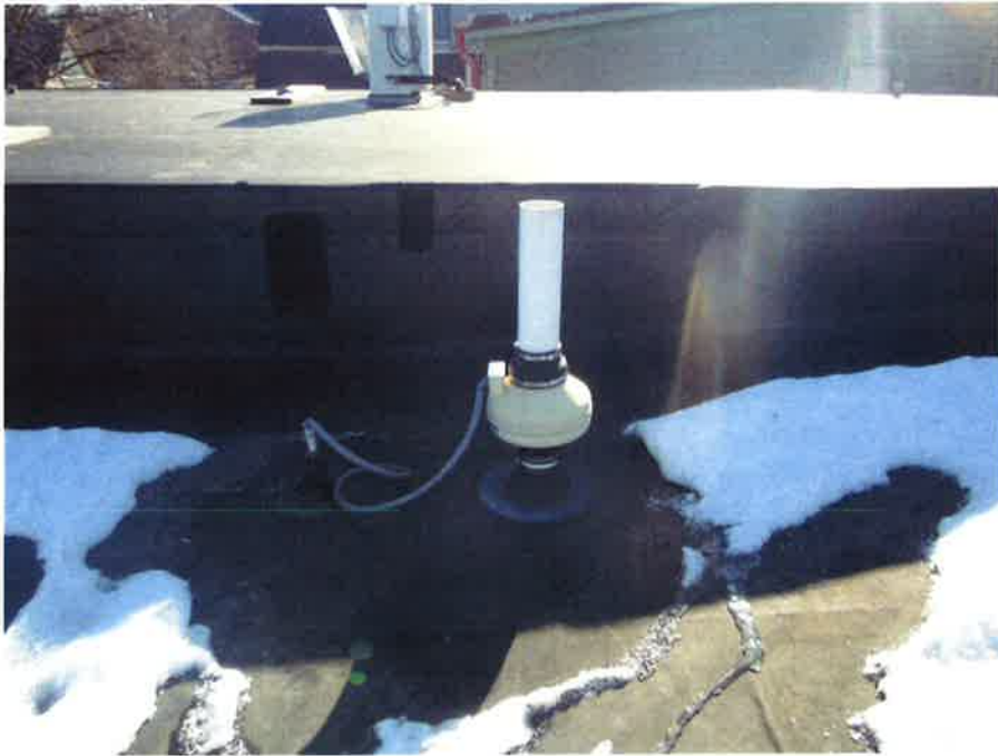
Photograph 2 – Southern SSV Mitigation Roof Fan
