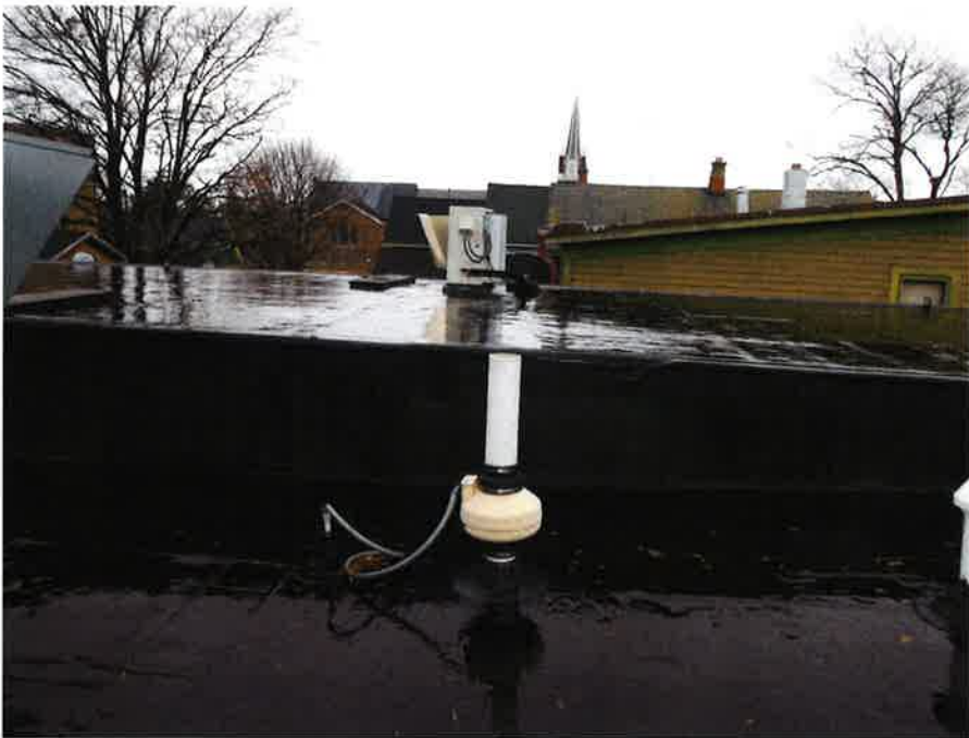
Photograph 2 – Southern SSV Mitigation Roof Fan
