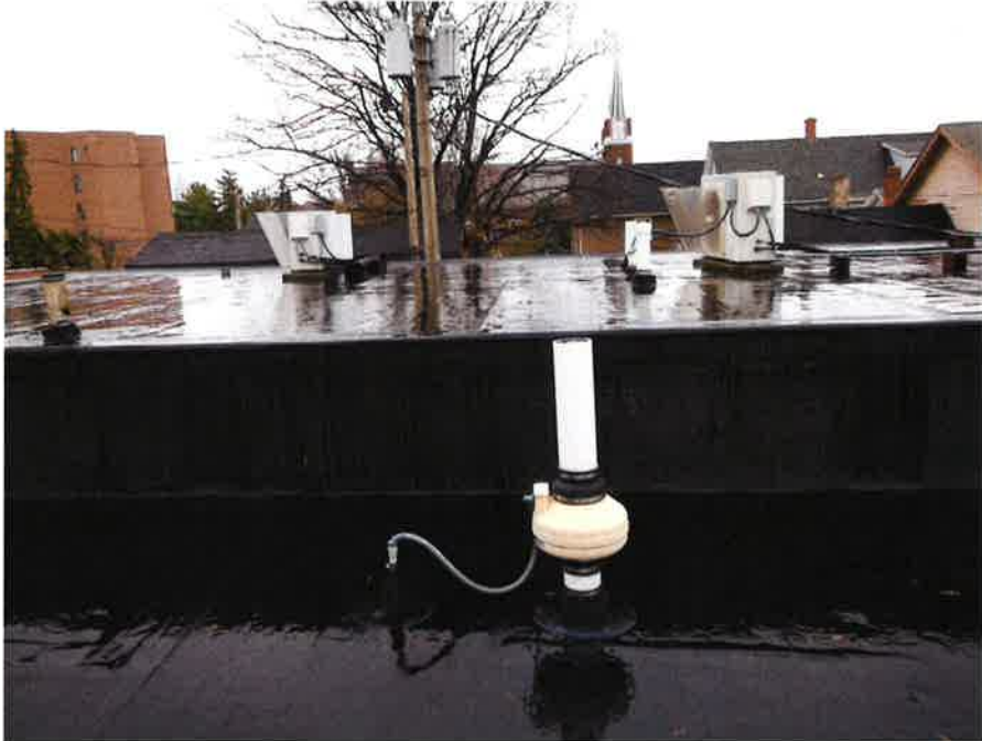
Photograph 1 – Northern SSV Mitigation Roof Fan
