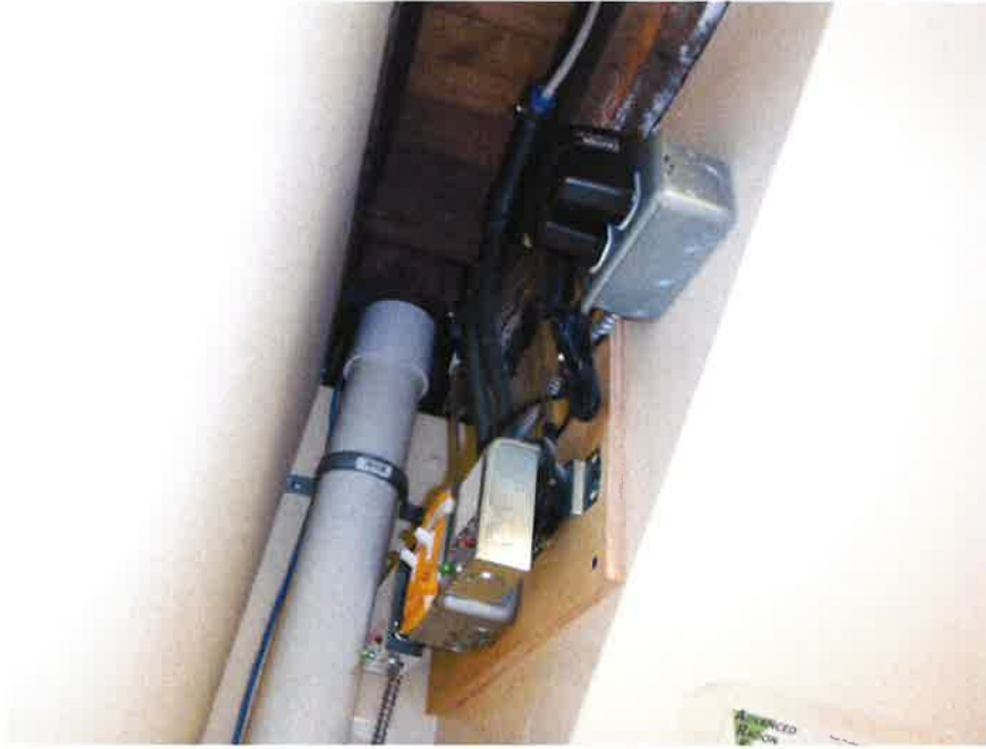
Photograph 11 – SSV Mitigation System Controls and Monitoring Equipment
