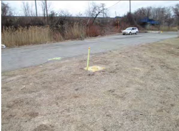
Photo 7: Asphalt cover and wetland buffer transition area in Site 2, Area 2B (taken facing southwest).
