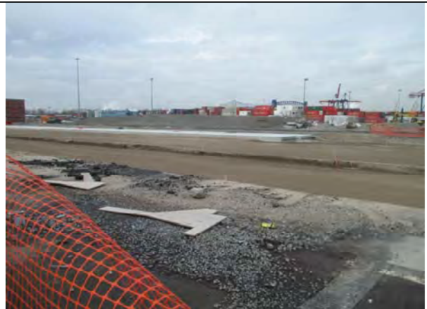
Photo 4: Construction for new rail tracks in Site 2, Area 2A taken facing southwest.
