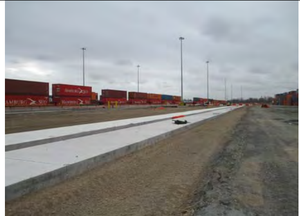
Photo 8: Excavation area for rail tracks in Site 2, Area 2B (tacking facing northwest).
