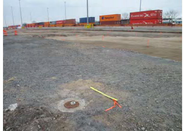
Photo 12: PRW-10 taken facing northeast. Note excavation for railroad track installation in background.
