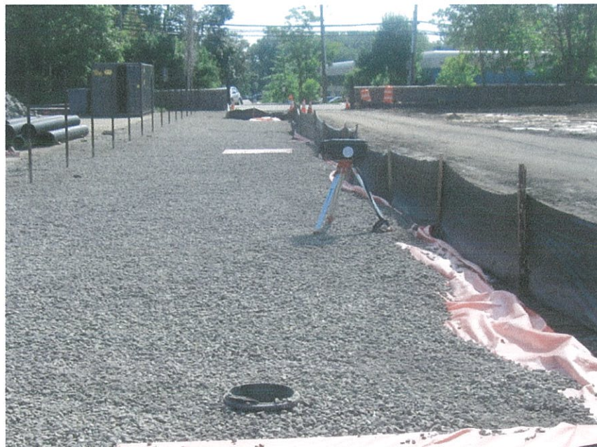
10. Downwind dust monitor near the catch basins.
