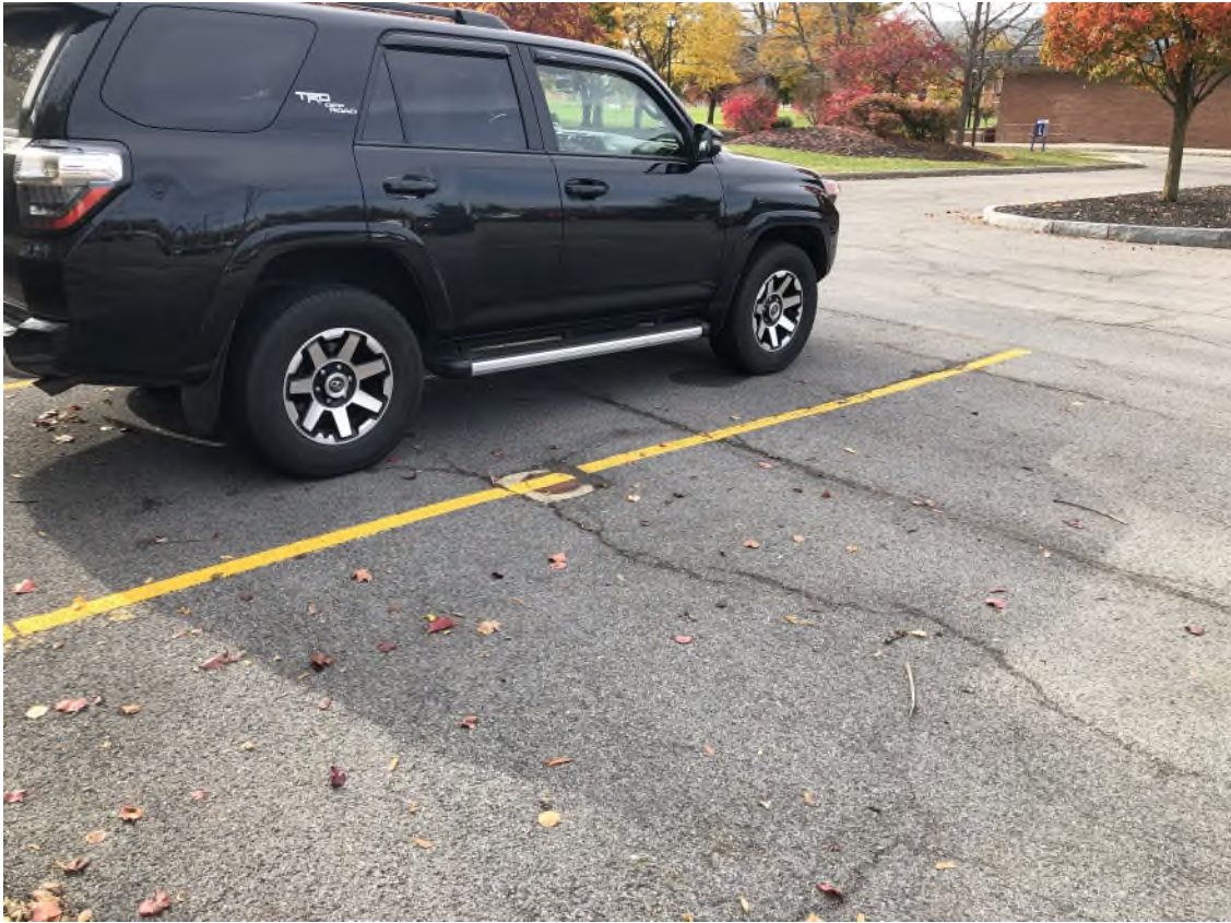
Asphalt cover near MW3, eastern portion of Parking Lot L - viewing southwest
