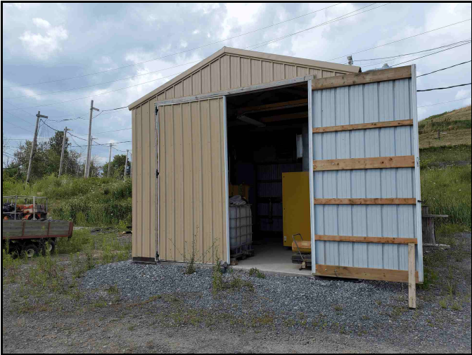
Odor neutralizing system in noise enclosure
