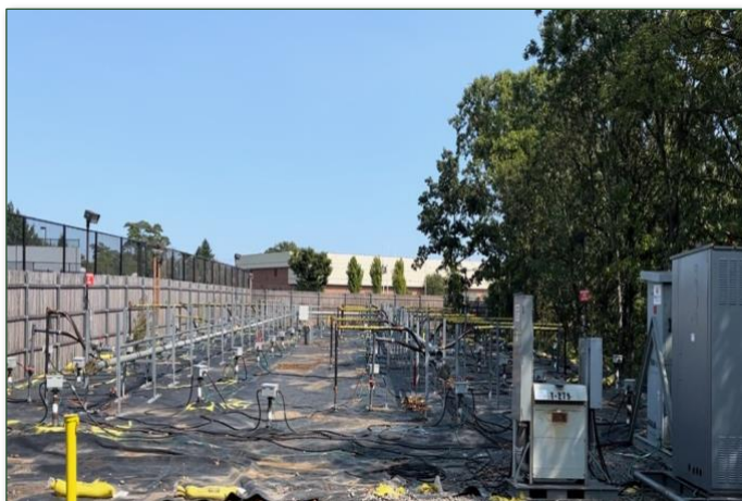
Thermal wells near the tennis courts
