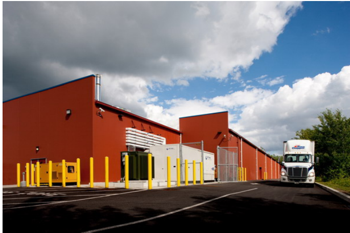
A 400-kW fuel cell (grey box) meets 85 percent of the energy needs of this Price Chopper supermarket in Albany. The installation reduces the building's carbon footprint by 71 tons, provides energy security for perishable items, and saves more than 4 million gallons of water each year. (Photo courtesy of UTC Power)
