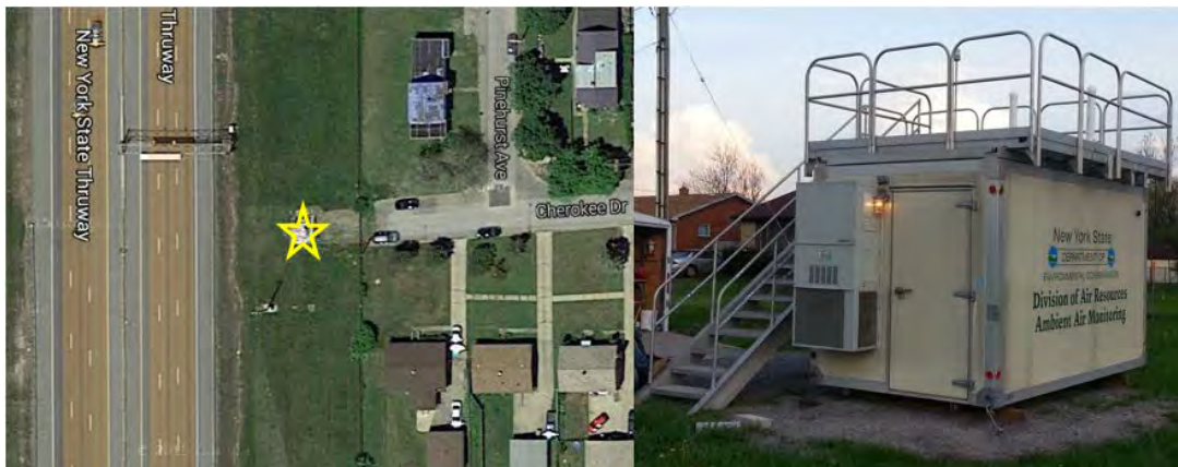
Figure 4. Buffalo Near-road Monitoring Station
