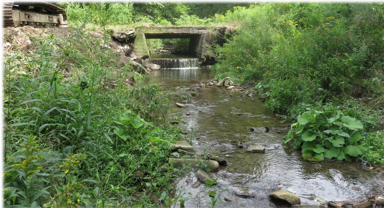
Figure 1. Culvert on Indian Creek impassable to fish prior to construction of a rock riffle.
