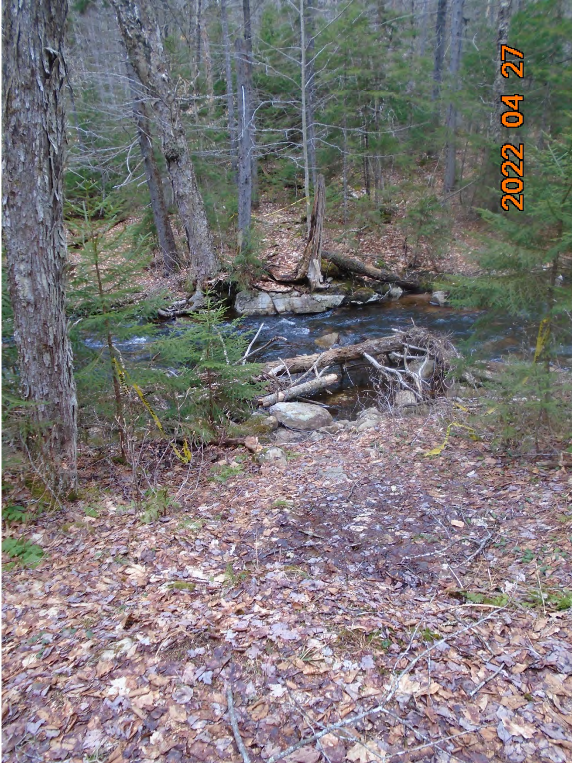
Looking north at the crossing from the southern bank following the removal of the bridge.
