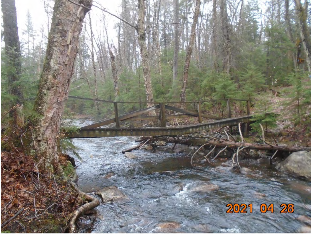
Looking east at the bridge from the northern bank just prior to its removal
