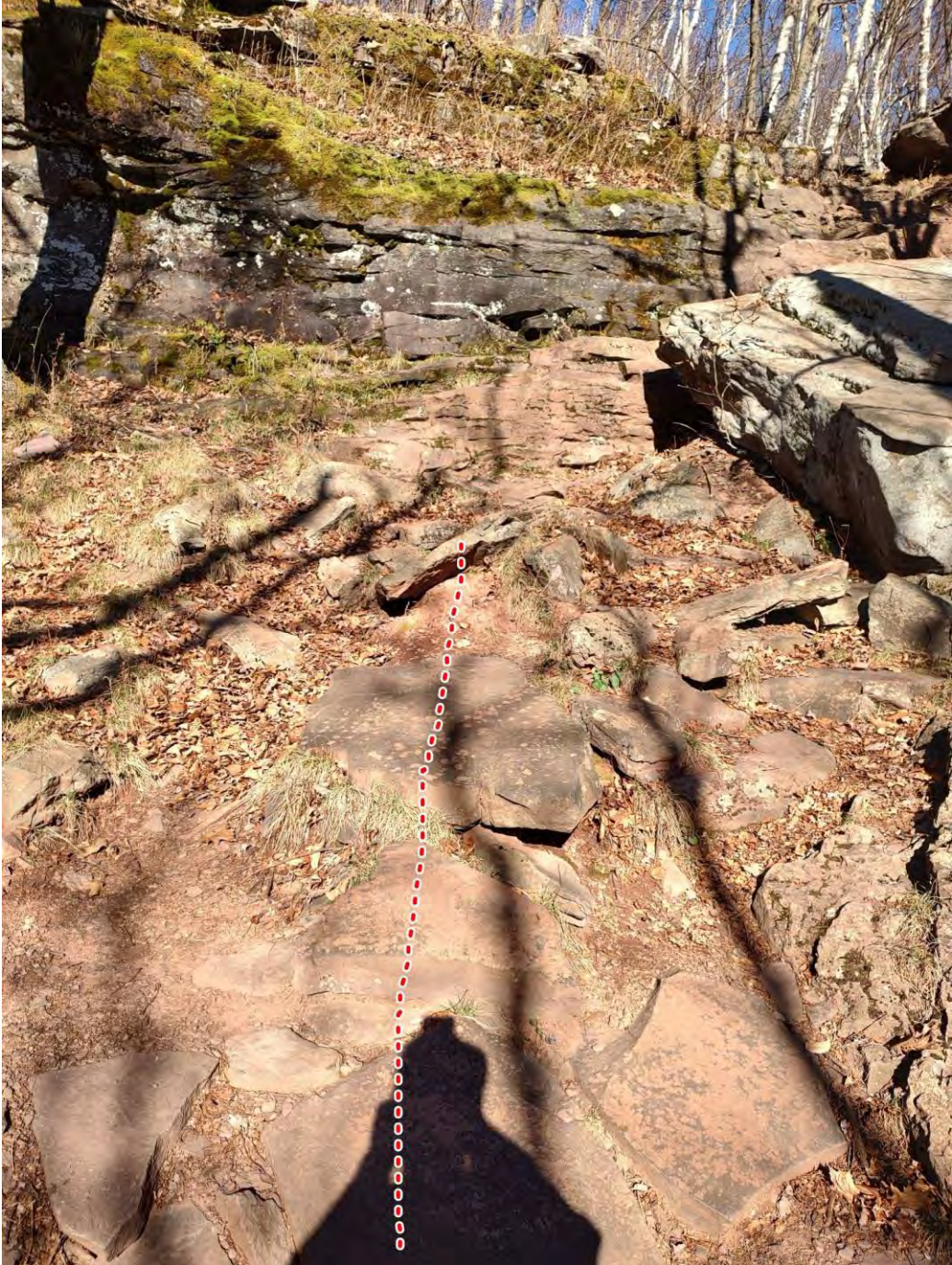
Uppermost Staircase: Should be completely rebuilt and extended
