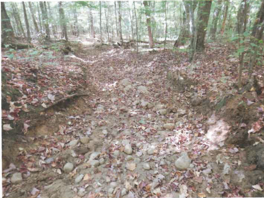
The hill on Icicle Trail is eroded, and loose cobbles provide unstable footing for equestrian use.
