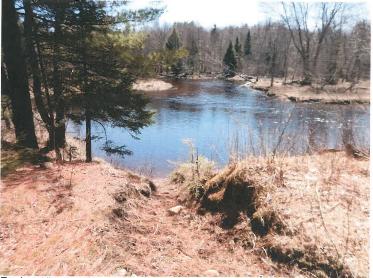
Erosion at the equestrian water access on Burnt Creek Trail
