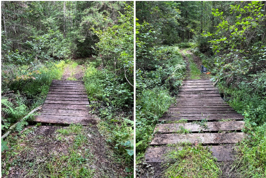
While not readily apparent from pictures, the stringers have failed in the center of the bridge, and the bridge now rests in the crossing (an inlet to Pine Lake). Existing bridge facing east (left), existing bridge facing west (right)
