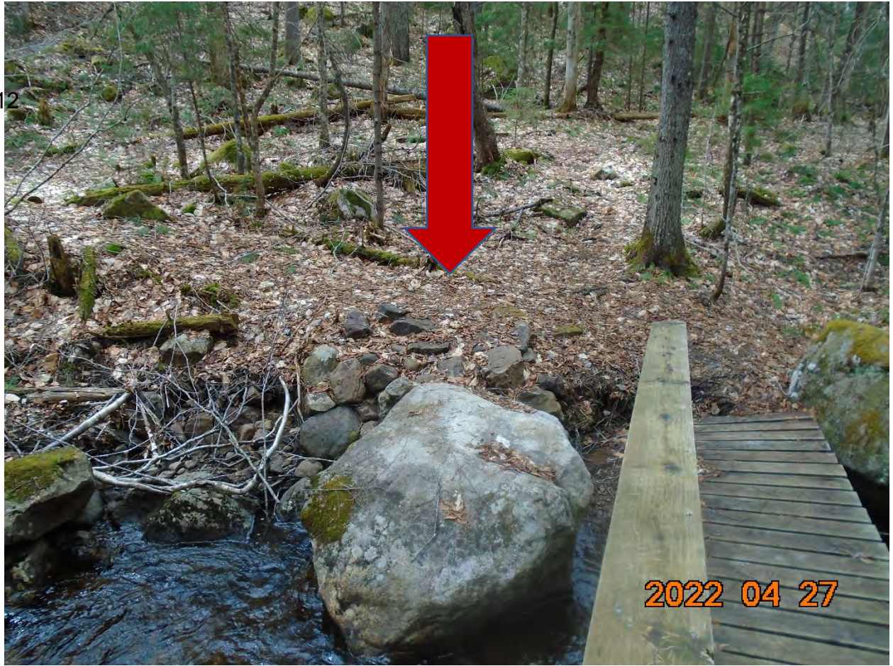
Looking at the western bank from the bridge. The red arrow denotes where the sill and end of the new bridge will be installed.
