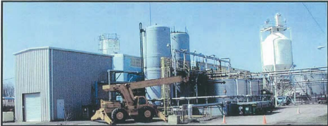
PHOTO 6 – AQUEOUS WASTEWATER TREATMENT FACILITY (T01)
