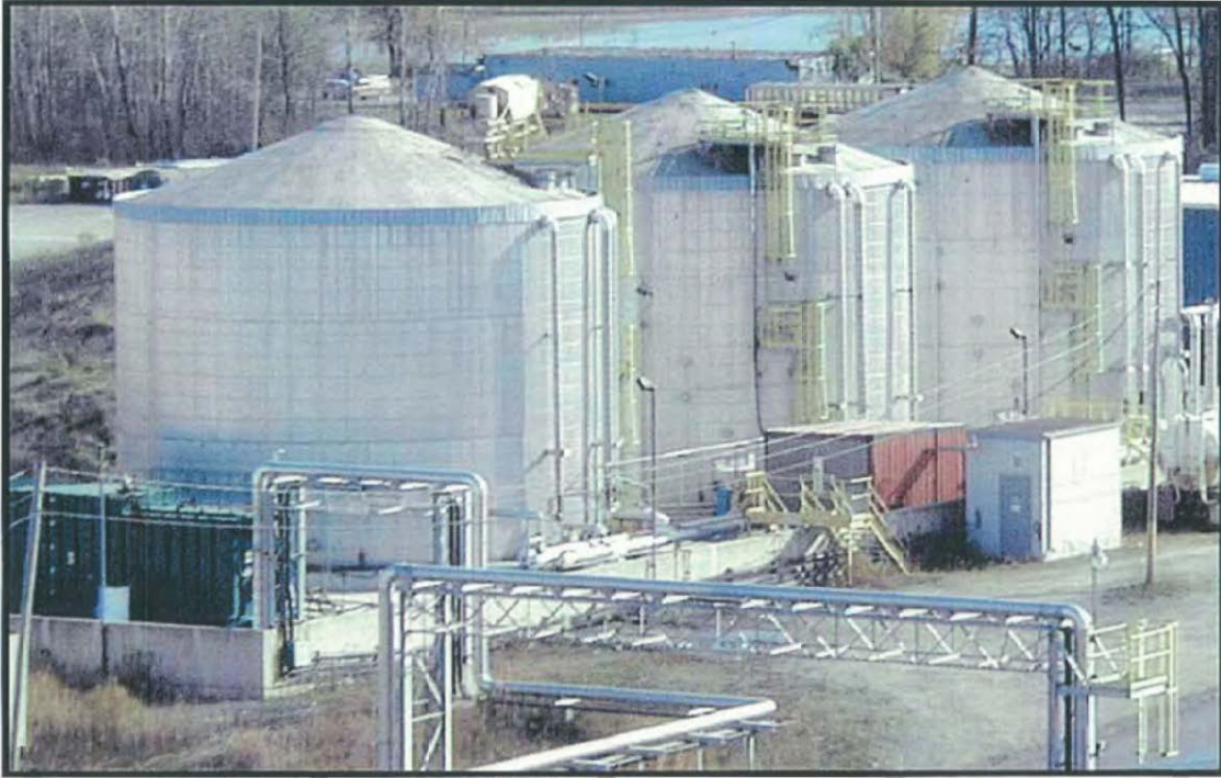
PHOTO 8 – LEACHATE TANK FARM (S02)
