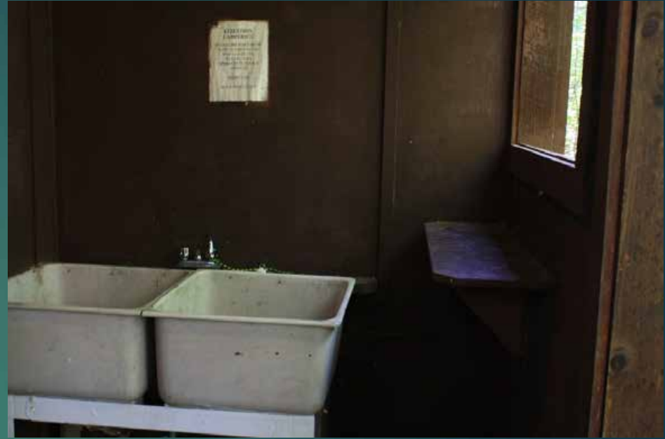
Comfort Station Slop Sink
