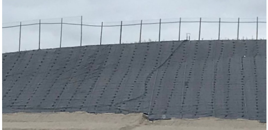
Odor neutralizer distribution lines installed by WM during 2020-2021. Photo: NYSDEC
