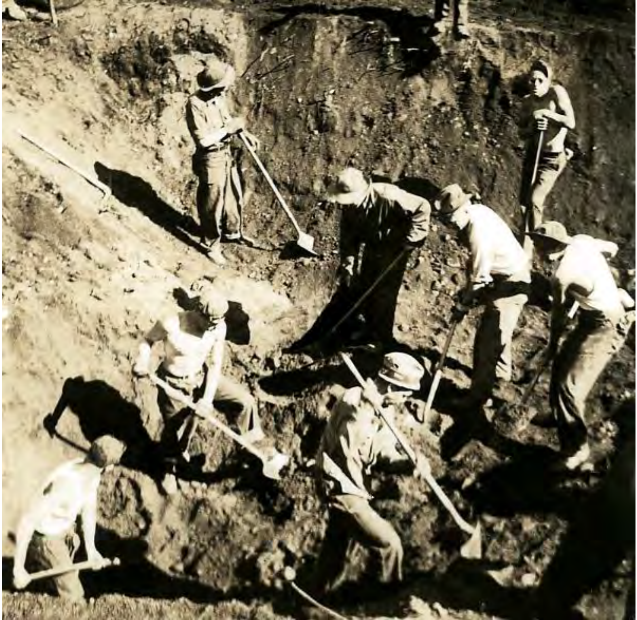
Whiskey Flats State Forest – RA 2 Proposal L, Town of Hopkinton Digging a waterhole along the west side of what is now the Hayden Rd Built by CCC Camp S-134 (Pierrepoint) in 1936. Foreman Clawson.
