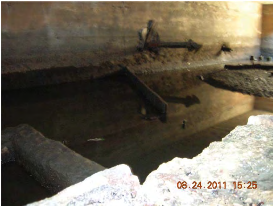
Picture #9- Inside Oil Skimmer looking NW at pipe penetrations and internal baffles
