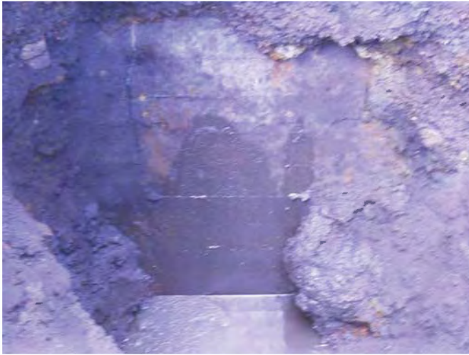
TP-14 – groundwater encountered in test pit
