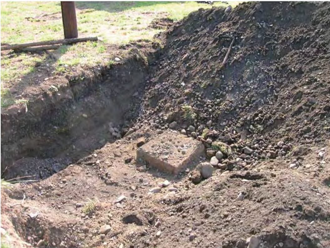
Picture #2- Oil Skimmer manhole uncovered
