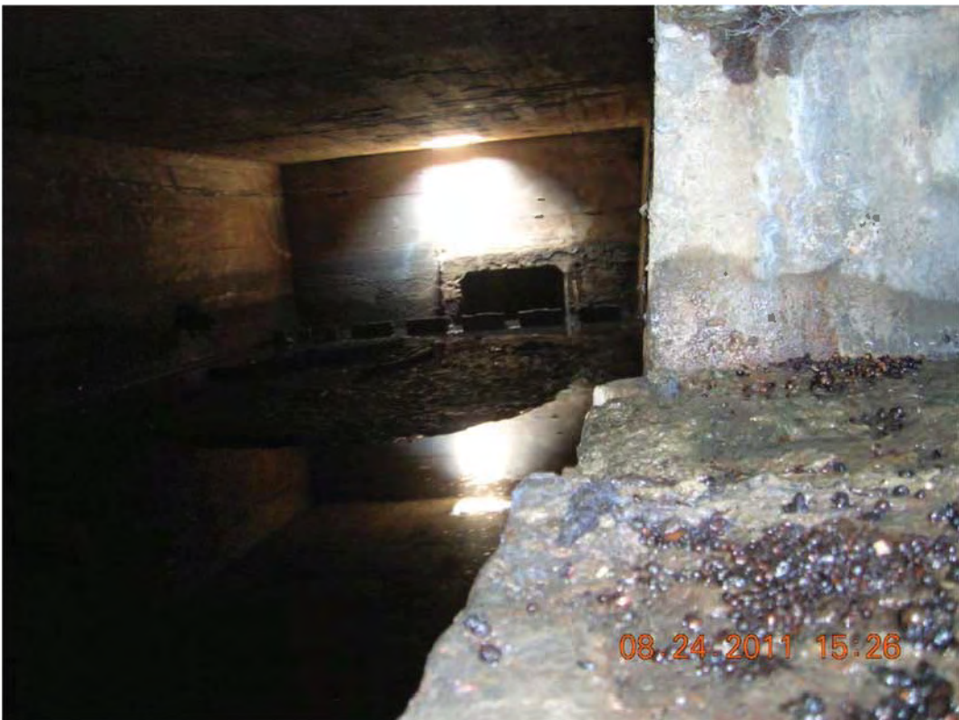
Picture #8- Inside Oil skimmer from Main Site Culvert looking east to ~5' wide culvert
