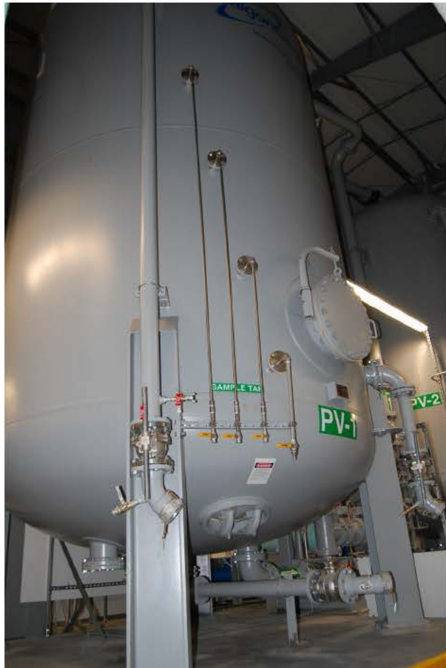
Figure 2: Steel vessel containing granular activated carbon (GAC).
