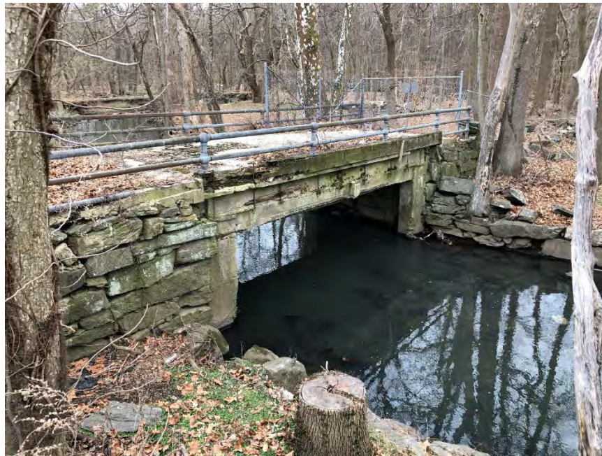
Figure 4-22: Looking downstream at pedestrian bridge inlet over Blind Brook. The bridge has been posted and fenced off on both sides to prevent passage.
