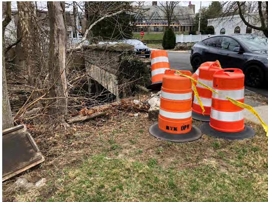
Figure 4-35: Looking at sidewalk damage and collapsed portion of the bridge parapet at the upstream bridge face
