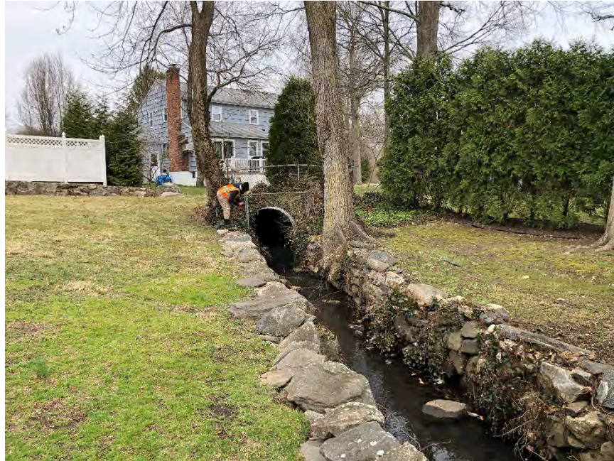
Figure 4-80: Looking upstream at the outlet of the culverts that run under Acker Drive. The stream is channelized behind the backyards of homes for most of its length as depicted.
