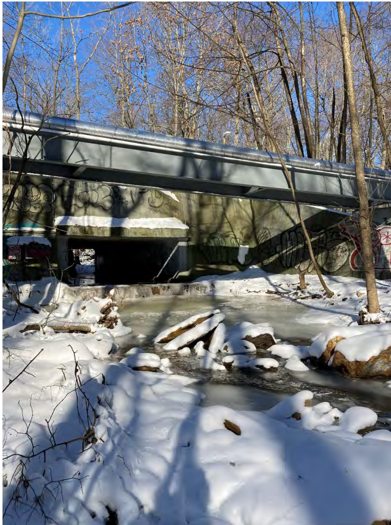
Figure 4-74: Looking upstream at the Salter Drive culvert. A water line for the SUNY Purchase College Campus Thermal Energy Storage Project runs on the downstream side of the structure.
