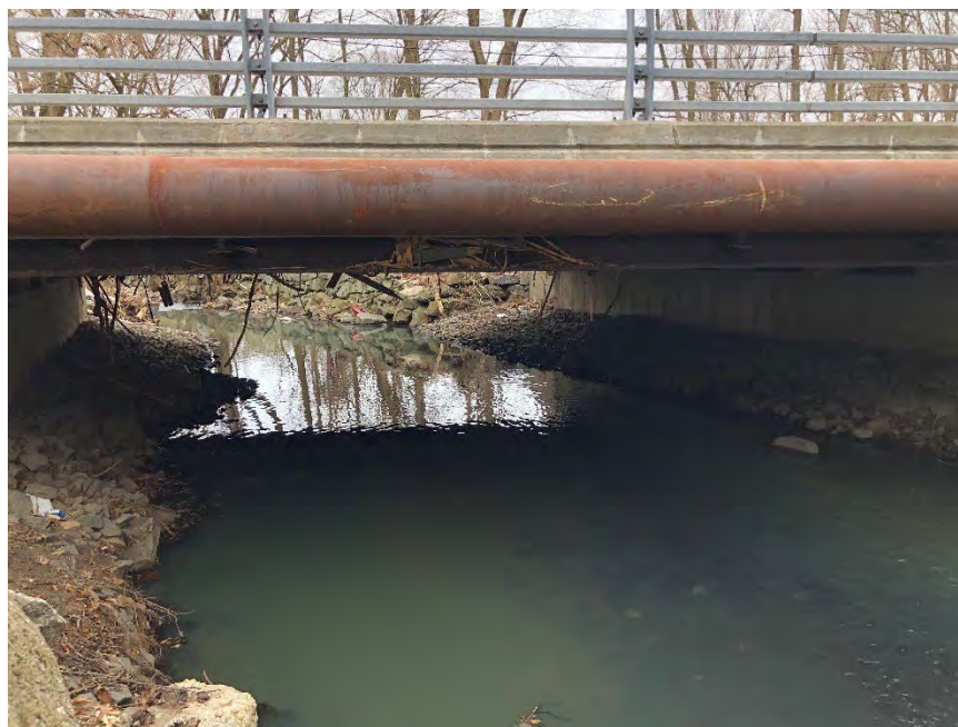
Figure 4-66: Looking downstream at the Westchester Avenue bridge over Blind Brook. A significant amount of woody debris is seen underneath the bridge deck, indicative of flood flows reaching the bridge's low chord.
