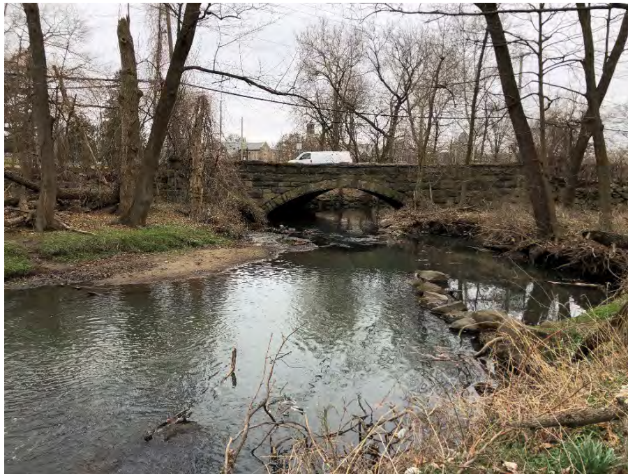
Figure 4-14: Looking downstream at the Boston Post Road bridge inlet over Blind Brook
