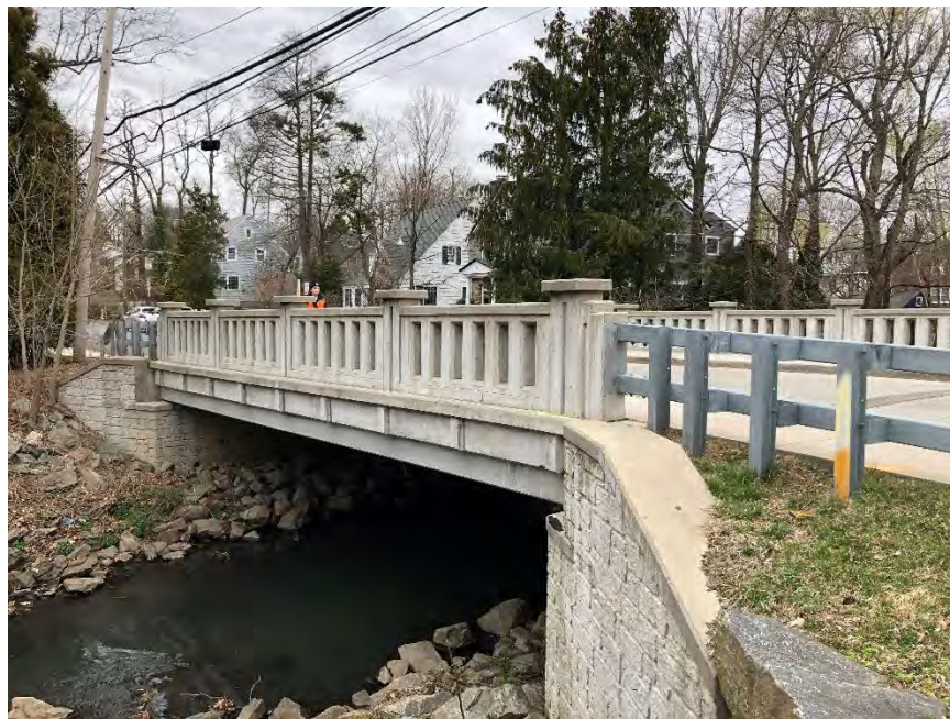
Figure 4-33: Looking upstream at the Central Avenue bridge. The crossing at this location was replaced in 2013 with a larger span bridge.
