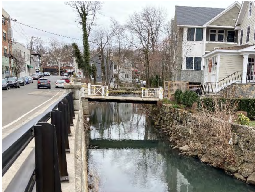
Figure 4-38: Looking downstream at the walled-in section of Blind Brook and the private pedestrian bridge that spans over it. The bridge is missing portions of the guardrail, and yellow caution tape has been added around the structure.
