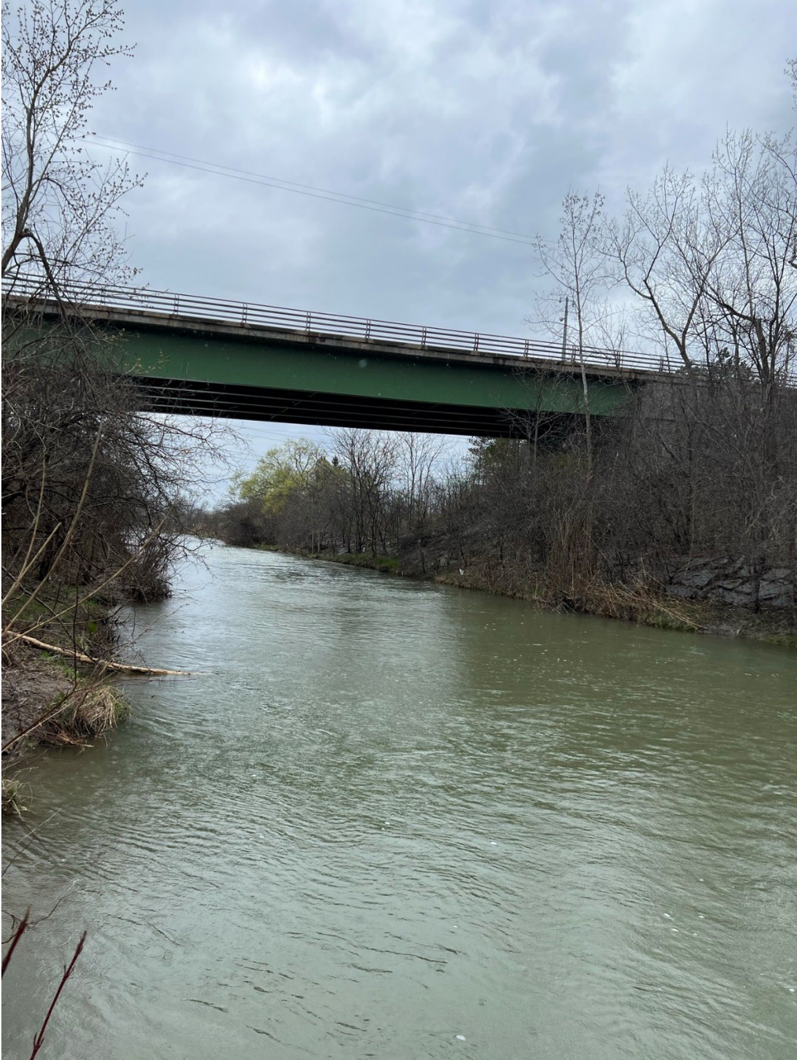
Photo D-9. Looking upstream toward the Kinne Road bridge from the right bank.
