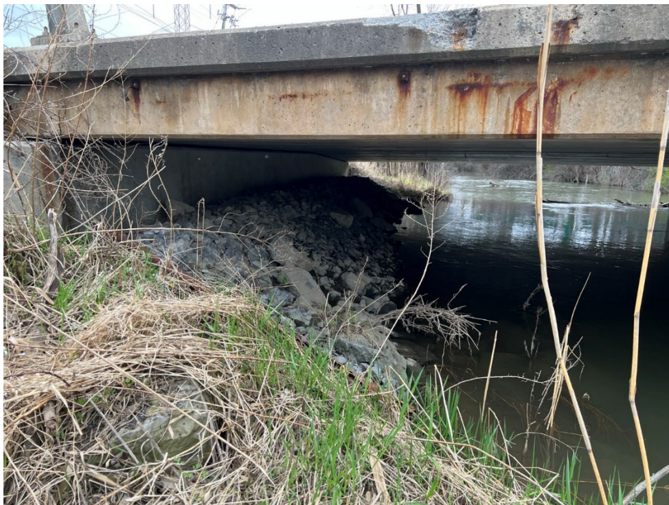
Photo D-6. Looking downstream standing at the upstream face of the NYS Rt. 290 bridge.
