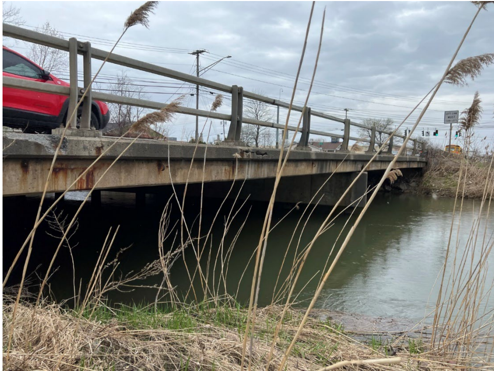
Photo D-5. Looking across the downstream face of the NYS Rt. 290 bridge, taken from just downstream of the bridge on the right bank. Photo taken 4/21/22 by GSE.
