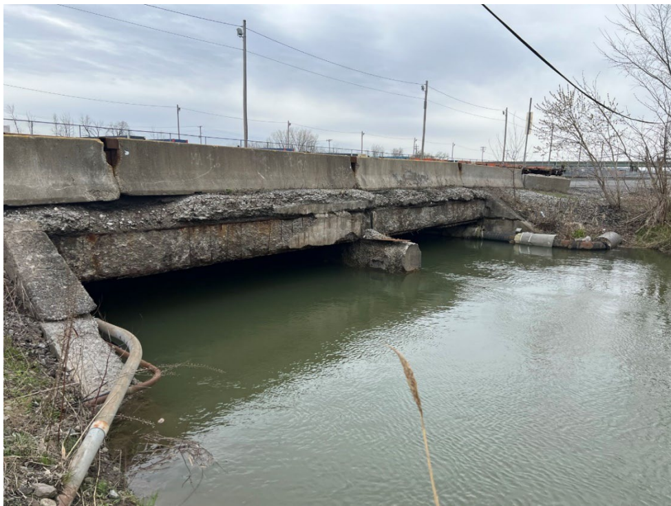
Photo D-2. Looking across the downstream face of the CSX railroad crossing.
