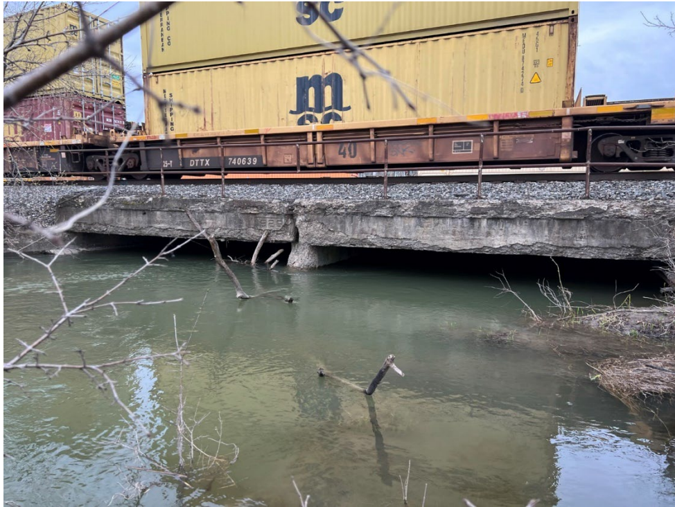
Photo D-3. Looking toward the upstream face of the CSX railroad crossing from the right bank.
