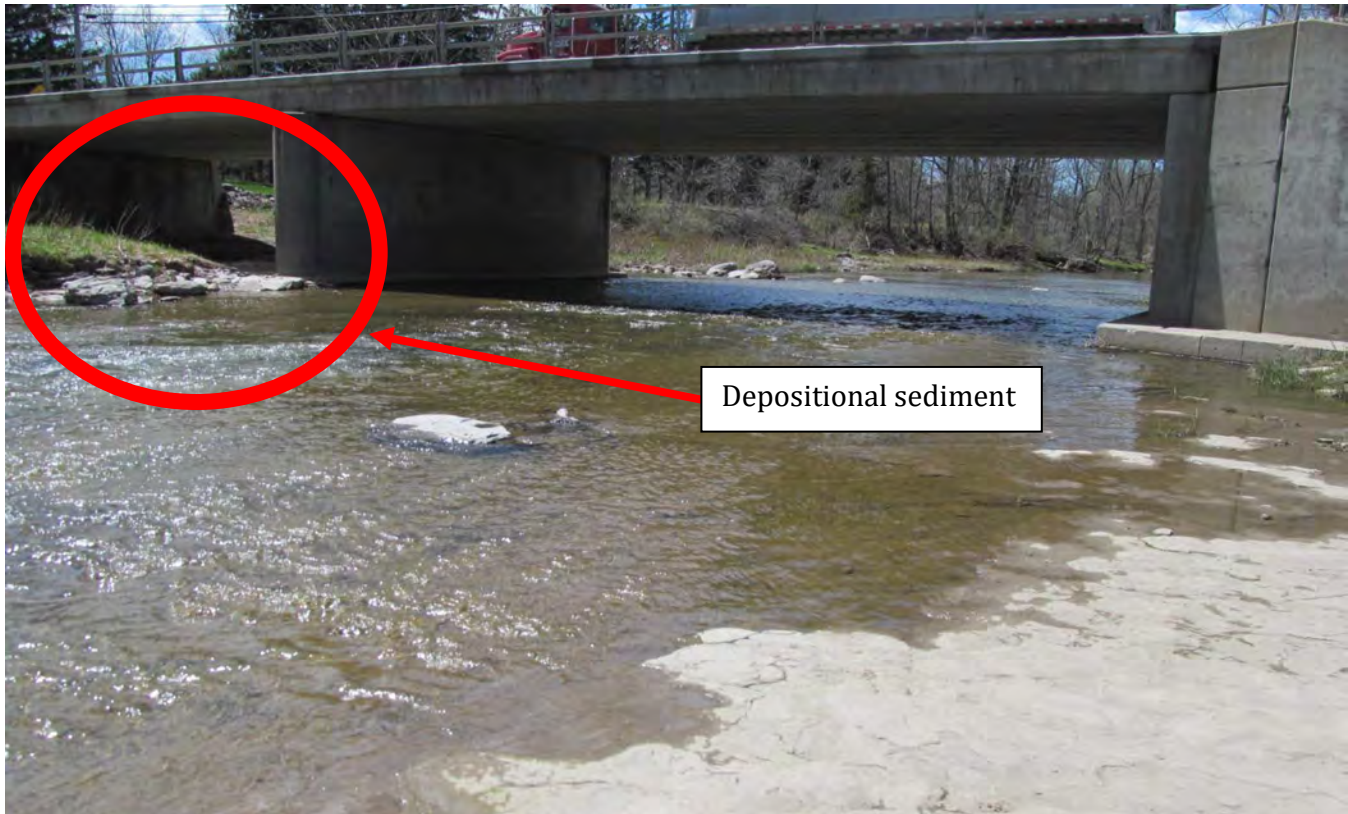
Figure 38. Depositional sediment underneath and in the vicinity of the Bowen Road Bridge at river station 645+61.
