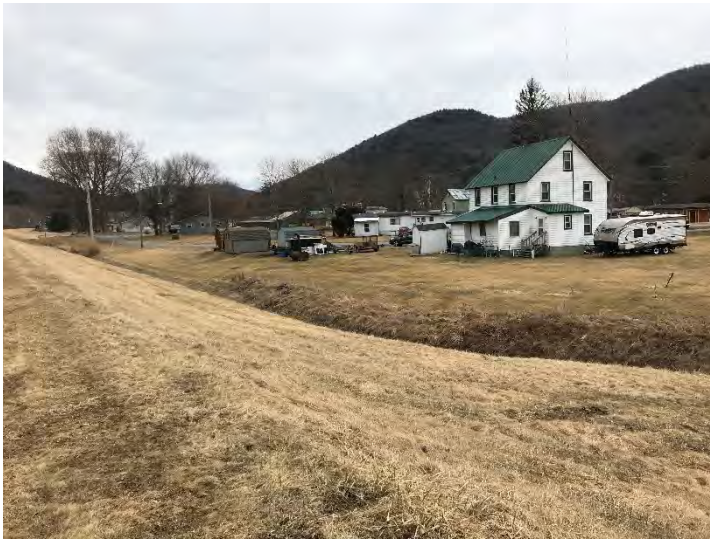
Photo 4-6 Levee in East Branch. View is from the levee crest, roughly to the southeast. Ponding area is out of frame to the photographer's right. EBDR is to the left. Outlet culvert with flap gate is behind photographer.
