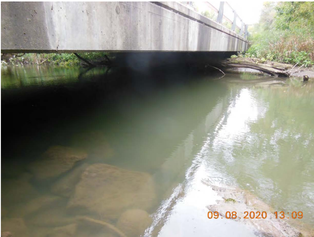
Photo D-4. Low Clearance under Plank Road Bridge
