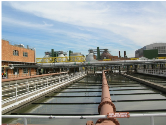
Final clarifier at Newtown Creek WWTP
