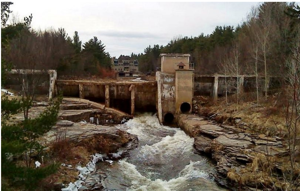
Figure 4-64 – LaSell Dam in 2007. The hydroelectric project was abandoned in the late 1950s – early 1960s and the penstocks and turbines sold for scrap. Note severe deterioration and evidence of alkali-silica reaction in the structural concrete and that one of the slabs in the primary spillway section had failed.
