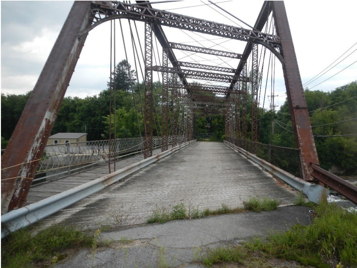
Figure 4-32: Out-of-service East Street bridge in the Hamlet of Mooers. Note deterioration of protective paint on the steel trusses and signs of corrosion.
