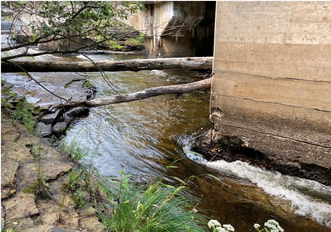
Figure 4-54: Upstream corner of McGregor Powerhouse. Note erosion of concrete and snagged woody debris.
