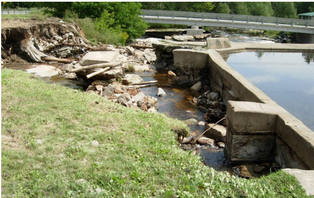
Figure 4-62: Damage to McGregor Dam on North Branch Great Chazy River due to overtopping in August 2010. Canaan Road bridge is in background. Photo is provided by Clinton County Emergency Services.
