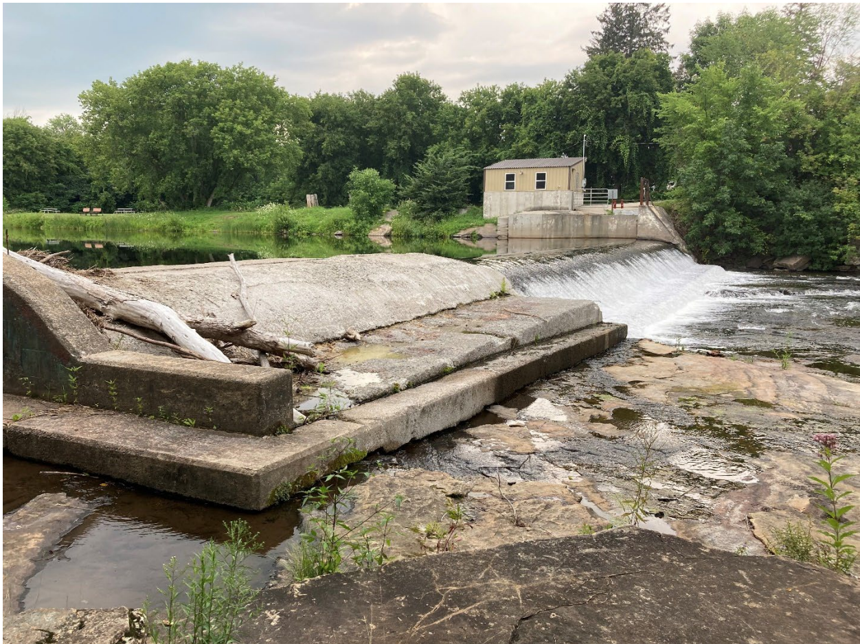
Figure 4-33: Mooers Dam. Fire suppression pump station is in background. Note seeps along concrete apron contact with bedrock in foreground.
