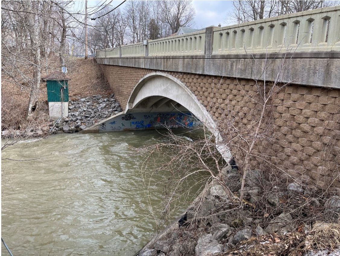
Figure 7-10. N Main Street/NY-65 bridge and a USGS gage station, Honeoye Falls, NY.
