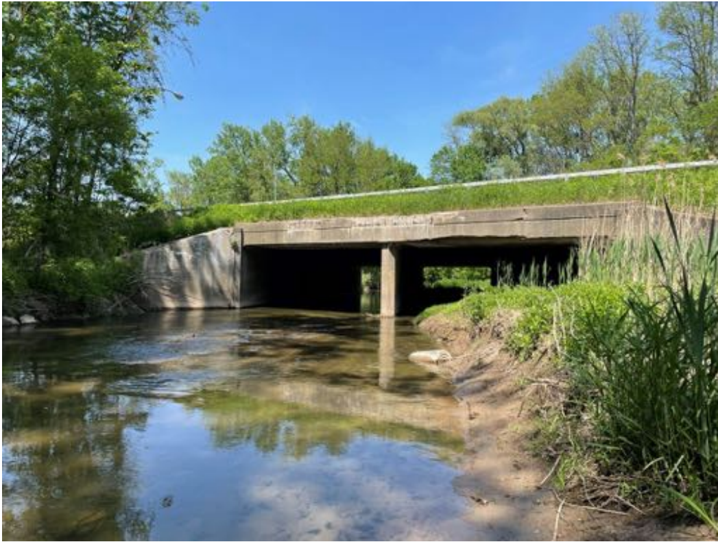
Photo D-7. Upstream Face of Interstate 490
