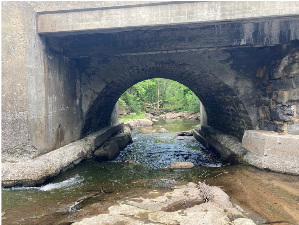
Figure 4-20: NY-22 bridge, looking downstream. Note the additional contraction into the older masonry arch within the bridge; deterioration of concrete knee walls, and spalling, ASR, and exposed rebar in the new concrete superstructure.
