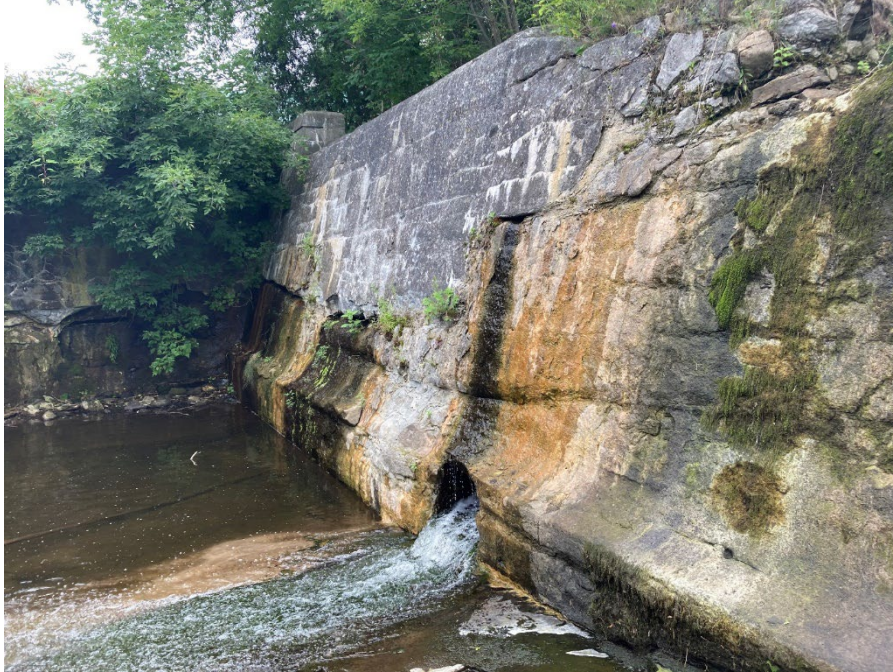
Figure 4-17: West Chazy Dam. Note major seep, ASR, cracks, and deteriorated concrete.
