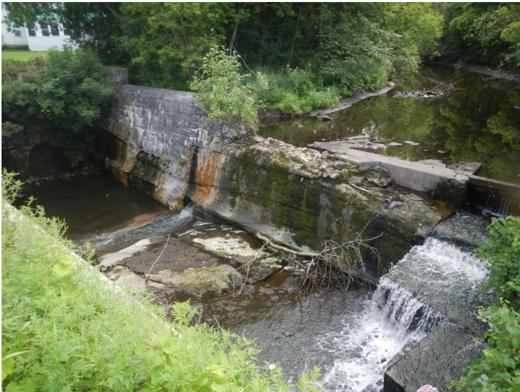
Figure 4-16: West Chazy Dam. Note significant seep at center-bottom of main dam section, evidence of ASR in the concrete, crack and deteriorated concrete, and vegetation growing in the concrete spillway.
