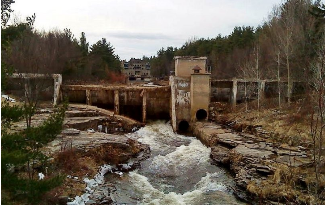
Figure 4-34: LaSell Dam on the Great Chazy River in 2007. The hydroelectric project was abandoned in the late 1950s – early 1960s and the penstocks and turbines sold for scrap. Note severe deterioration and evidence of alkali-silica reaction in the structural concrete and that one of the slabs in the primary spillway section had failed.
