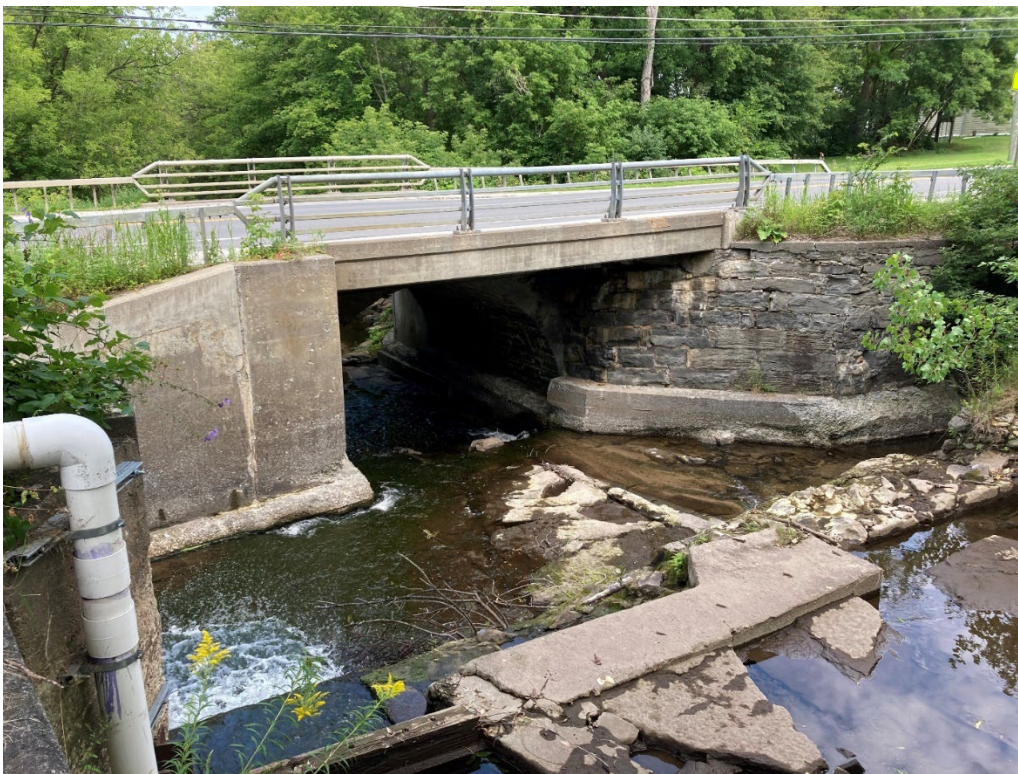
Figure 4-19: NY-22 bridge immediately downstream of the West Chazy Dam. Note significant contraction into bridge and dry hydrant in foreground as well as deteriorated spillway concrete.
