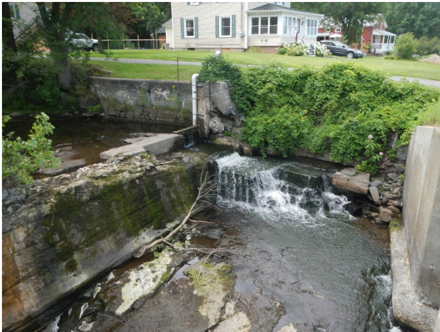
Figure 4-18: West Chazy Dam. Dry hydrant is visible near the center of the image, and the left abutment of NY-22 bridge is visible at right. Note deteriorated spillway crest and deteriorated left upstream training wall is leaning toward the river. The dam's left downstream abutment wingwall appears to be completely undermined (visible just to the right of vertical section of dry hydrant).
