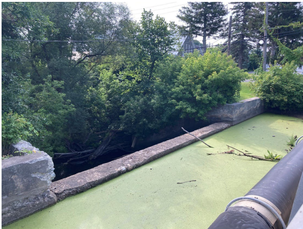
Figure 4-4: View of Little Chazy Dam primary spillway from US-9 bridge. Chazy Fire District building is visible in background, partly obscured by vegetation.
