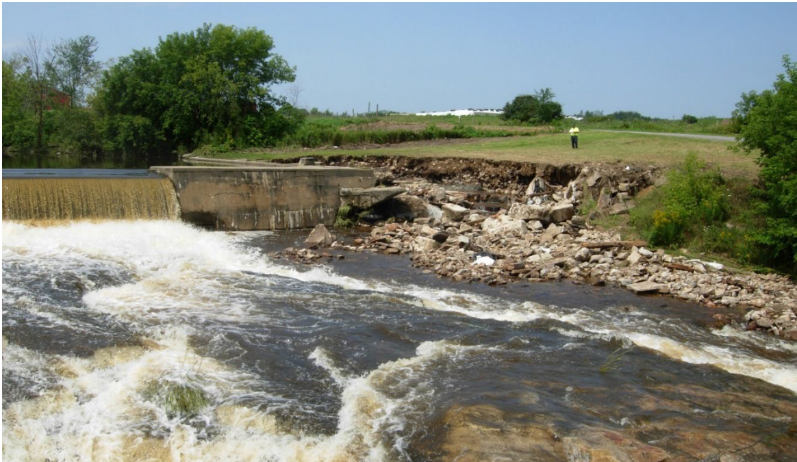
Figure 4-31: Overtopping during flooding in August 2010 caused washout of left embankment and undermining of abutment of McGregor Dam near the Canaan Road bridge in Ellenburg Depot. Photo provided by Clinton County Emergency Services.
