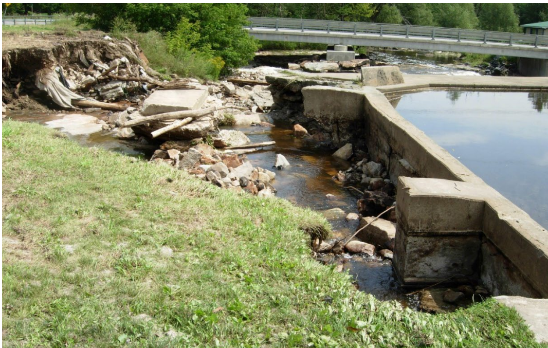
Figure 4-32: Damage to McGregor Dam on North Branch Great Chazy River due to overtopping in August 2010. Canaan Road bridge in background. Photo provided by Clinton County Emergency Services.
