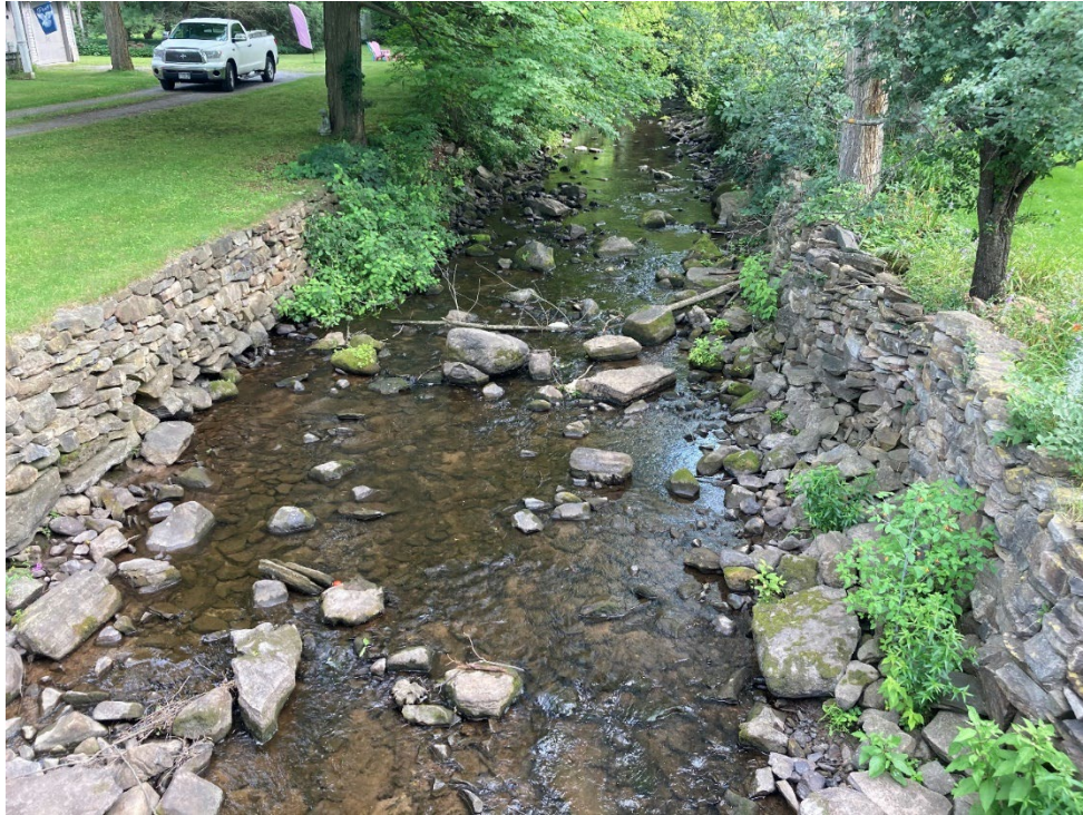
Figure 4-22: Confined and entrenched channel immediately upstream of the West Church Street bridge
