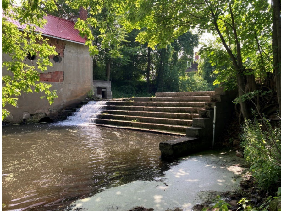
Figure 4-6: The W.H. Miner Dam #2 in West Chazy. Note deteriorated concrete spillway and powerhouse building.
