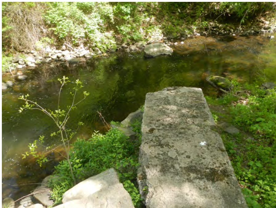
Figure 4-32 Breached Dam Located Approximately 4,000 Feet Downstream of Sky Meadow Road Crossings
