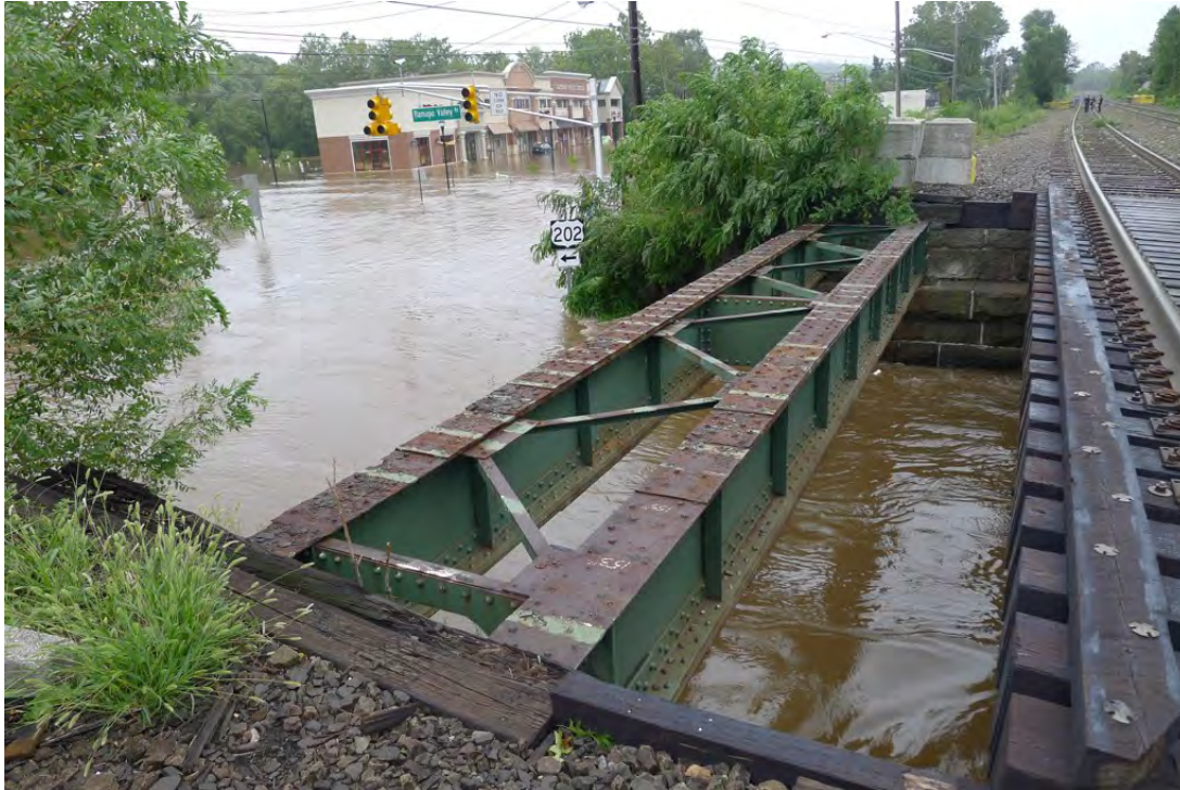
Figure 4-8A: US-202 underpass at Norfolk Southern Railroad, 550 feet north of the Mahwah River, during Tropical Storm Irene in 2011. Floodwaters are several feet deep on the roadway. Business park shown in Figure 4-8 is visible in background.
