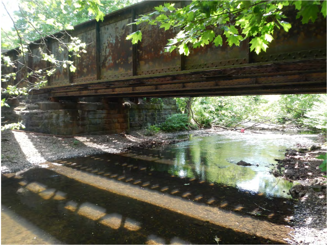
Figure 4-4: Norfolk Southern Railroad crossing of the Mahwah River in New Jersey. View looking downstream.
