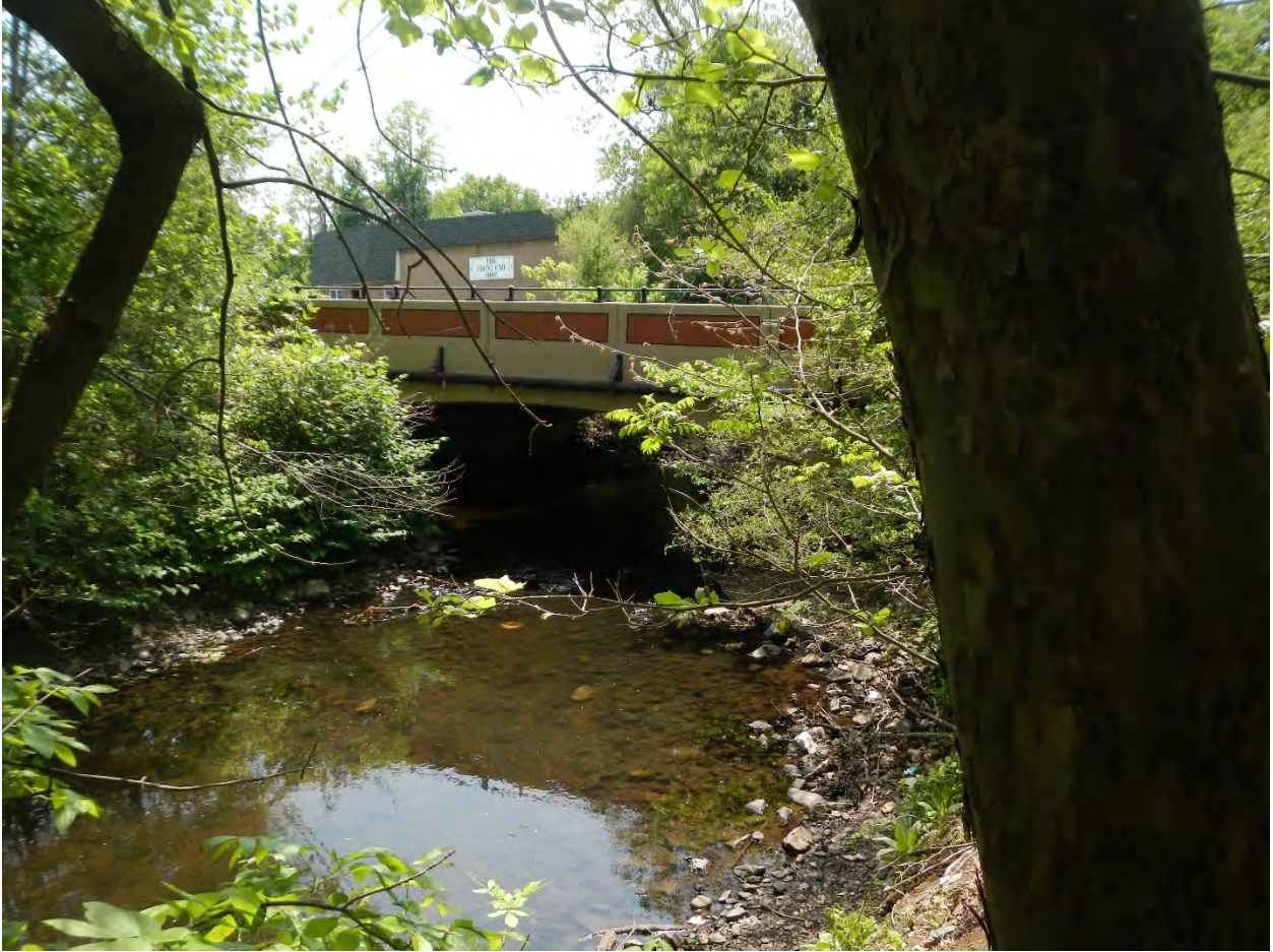
Figure 4-3: Franklin Turnpike crossing of the Mahwah River in New Jersey. View looking downstream.
