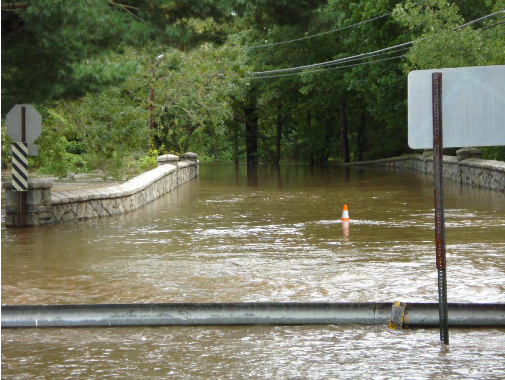
Figure 4-23 Montebello Road Bridge during Tropical Storm Irene. Photo courtesy of Rockland County.
