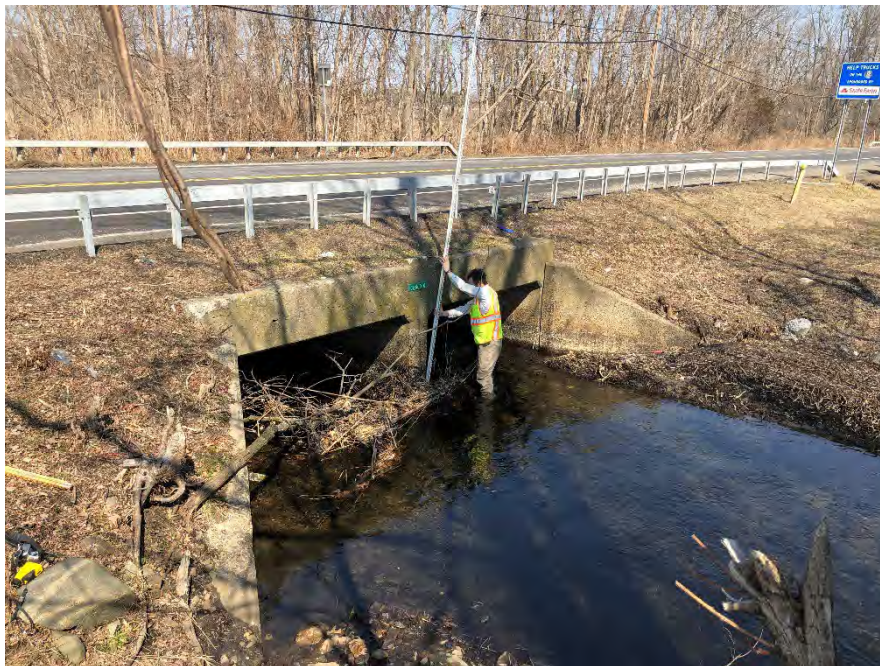
Figure 4-31: Inlet of Stream Crossing Structure under US Route 202
