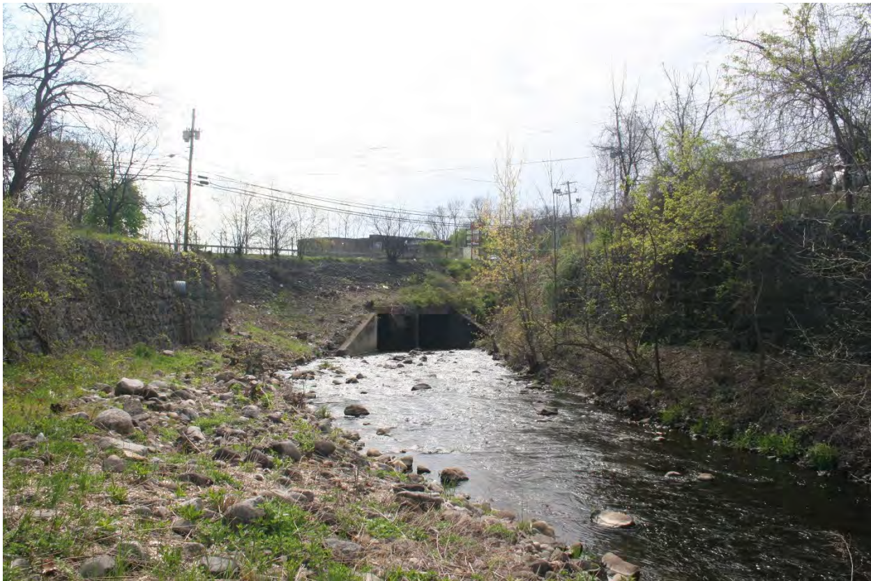
Figure 4-2: View Looking Downstream at Route 9W Culvert Crossing of Minisceongo Creek
