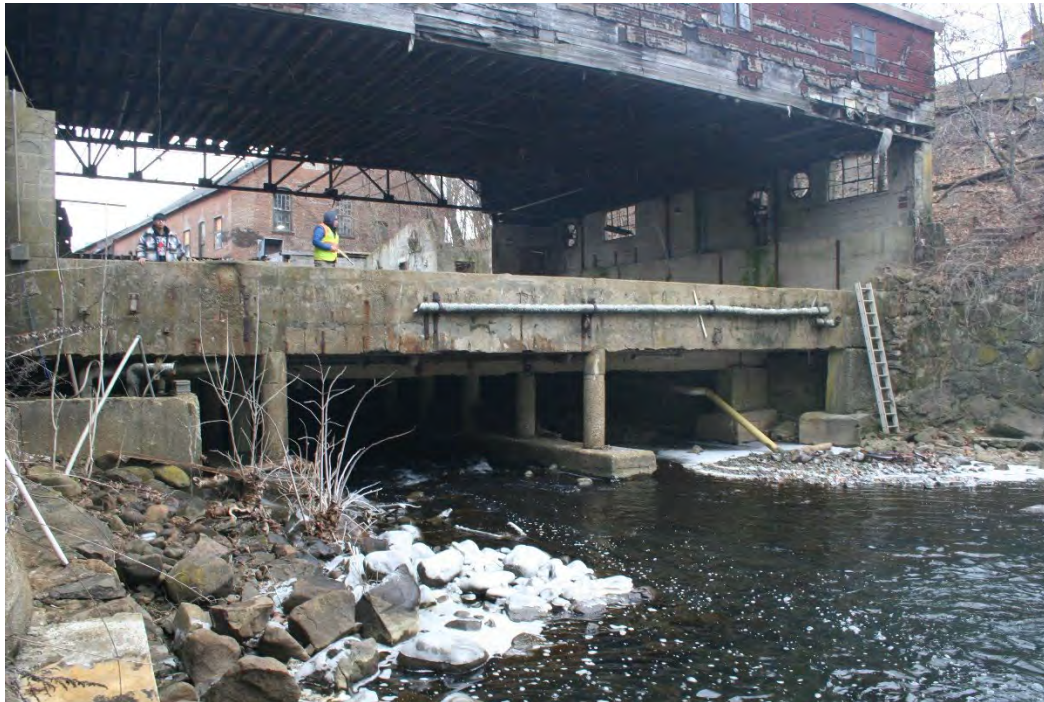
Figure 4-10: View looking downstream at upstream face of Building 26A at the GAIC just downstream of the Bridge Street dam. The elevated building 33A is also visible. Piers and other obstructions restrict flow and are prone to debris jamming.
