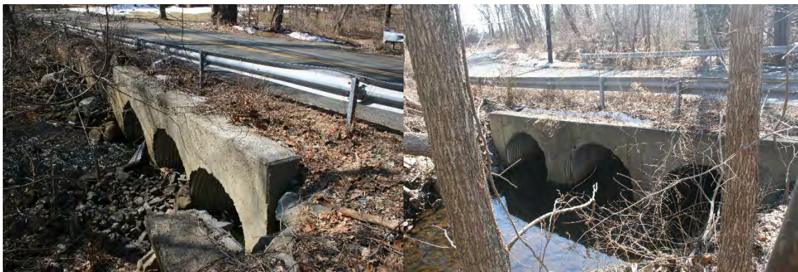
Figure 4-33: Inlet of Upstream Culverts (Left) and Outlet of Downstream Culverts (Right) on South Camphill Road
