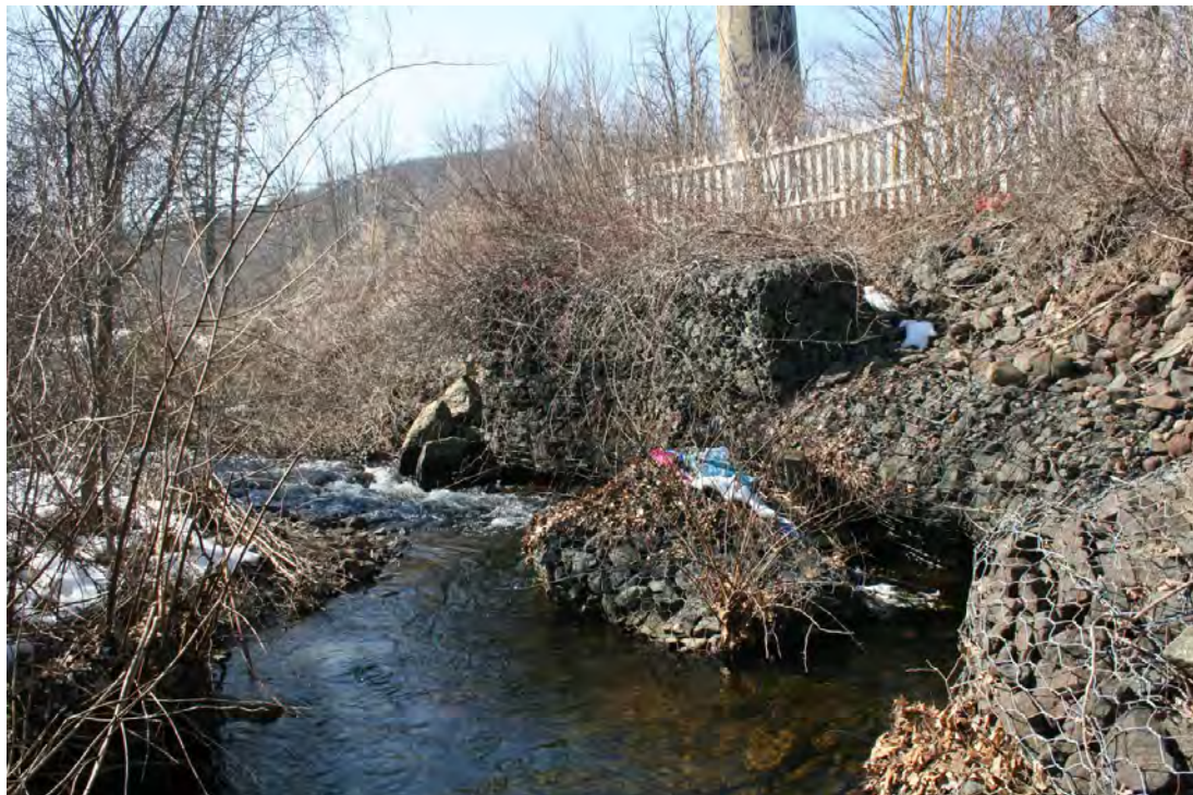
Figure 4-28: Gabions Falling into Minisceongo Creek Adjacent to Willow Grove Mobile Home Park
