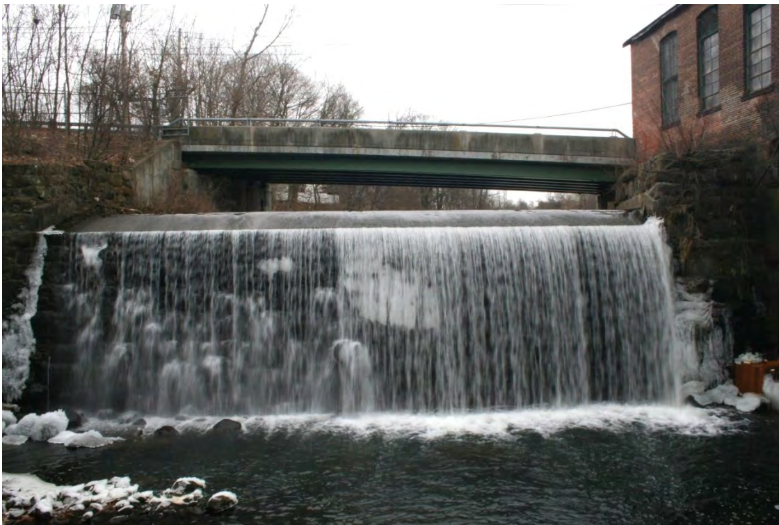
Figure 4-6: View of the Bridge Street dam from downstream. The Bridge Street bridge is visible just upstream.
