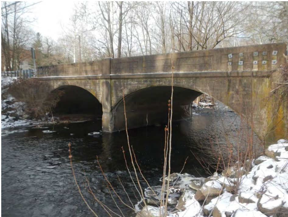
Figure 4-23: Older concrete arch bridge carrying Seven Lakes Drive over Ramapo River's right (westerly) channel
