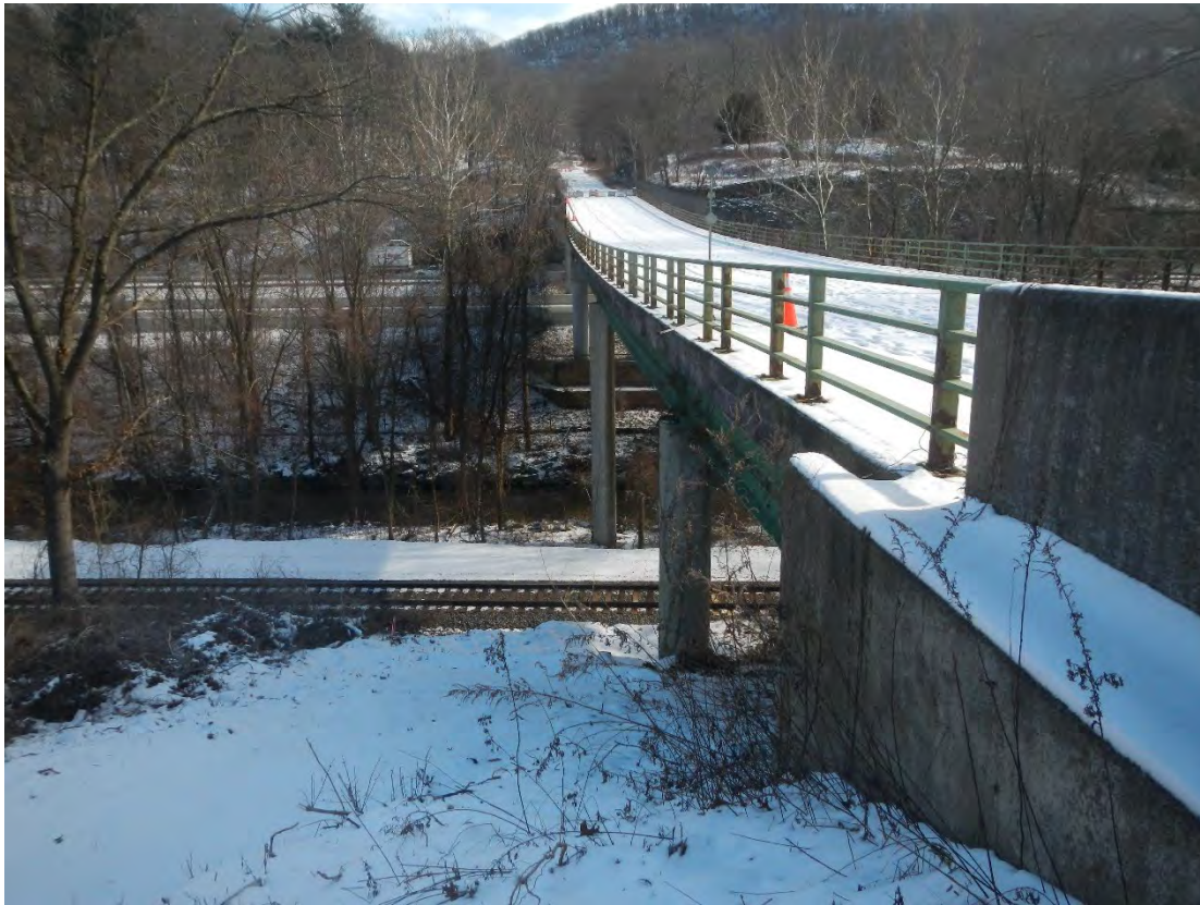
Figure 4-44: The Arden Valley Road bridge at STA 722+00 crossing the Metro-North/Norfolk Southern railroad, Ramapo River, and I-87
