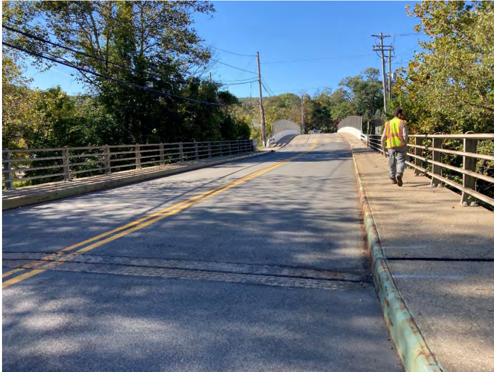
Figure 4-10: The Fourth Street bridge at STA 60+00, looking west. Bridge over the Ramapo River in center of image; bridge over I-87/NY-17 can be seen in the background.
