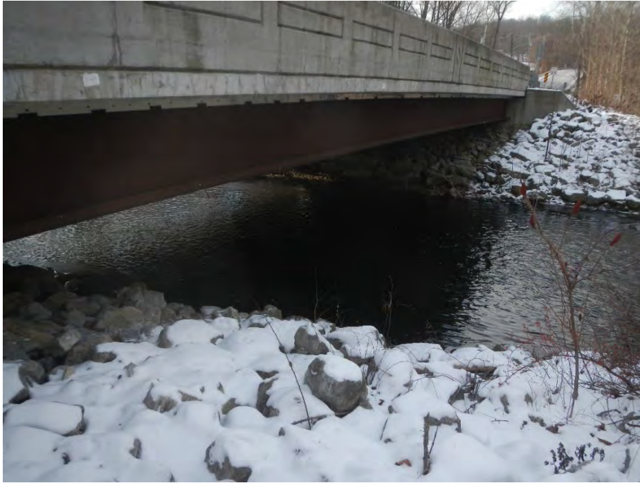
Figure 4-22: Newer steel beam bridge carrying Seven Lakes Drive over Ramapo River's left (easterly) channel
