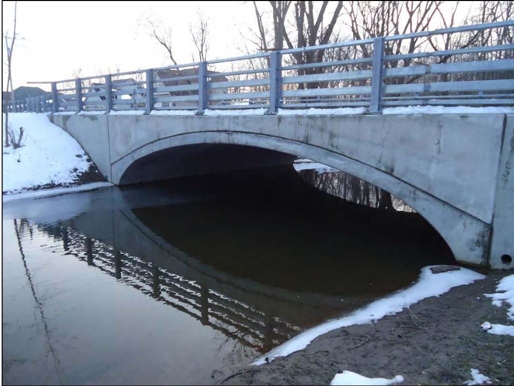
Photo D-12. Upstream face of Heise Road bridge crossing at Ransom Creek (2/17/2020)
