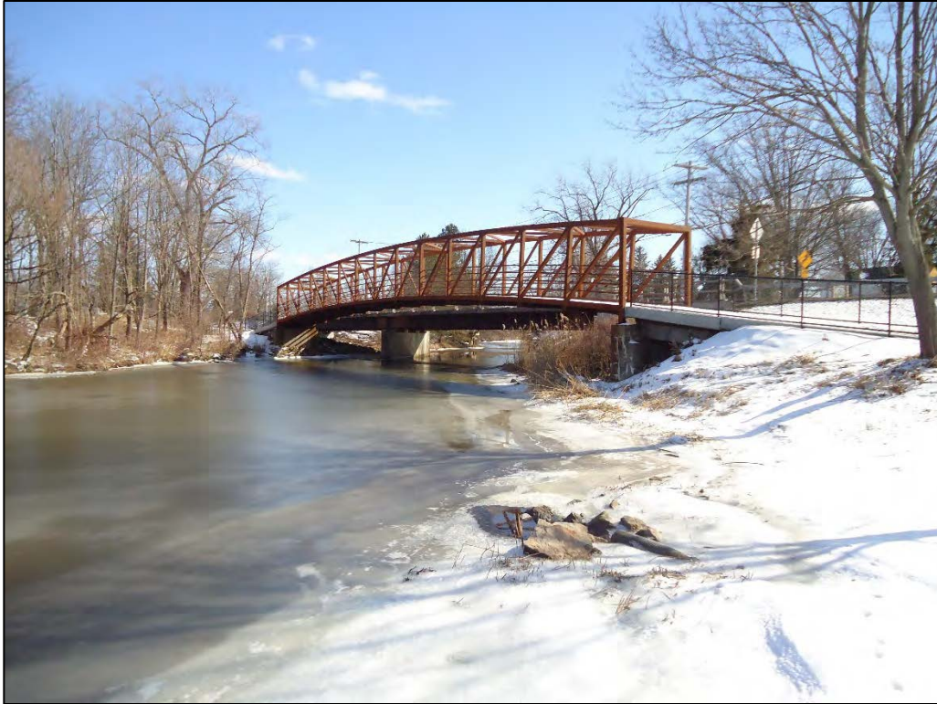
Photo D-1. Downstream face of bike path bridge crossing Ransom Creek near confluence with Tonawanda Creek (2/17/2020)
