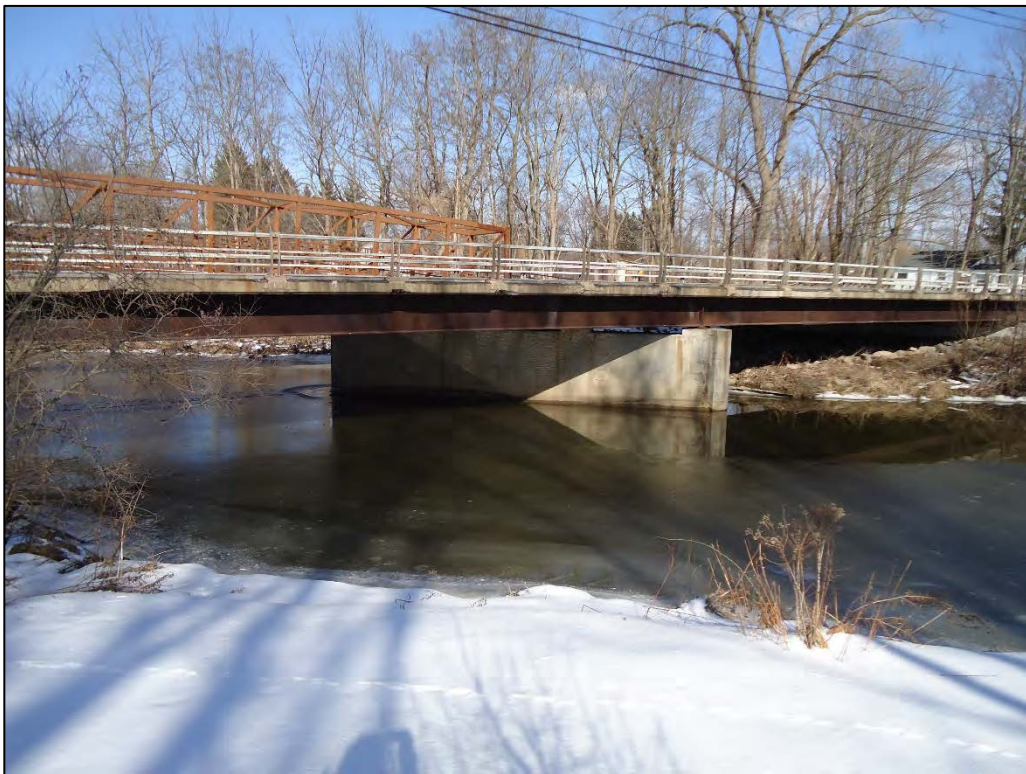
Photo D-2. Upstream face of Tonawanda Creek bridge crossing Ransom Creek near confluence with Tonawanda Creek (2/17/2020)
