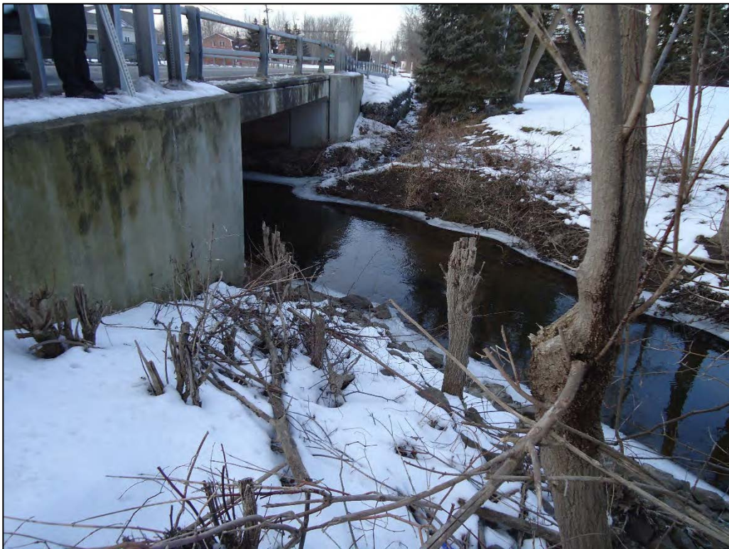
Photo D-11. Upstream face of Stahley Road bridge crossing at Ransom Creek (2/17/2020)
