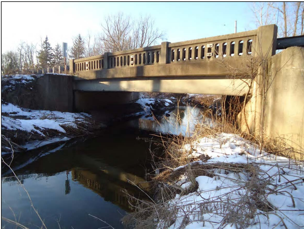
Photo D-9. Upstream face of County Road bridge crossing at Ransom Creek (2/17/2020)
