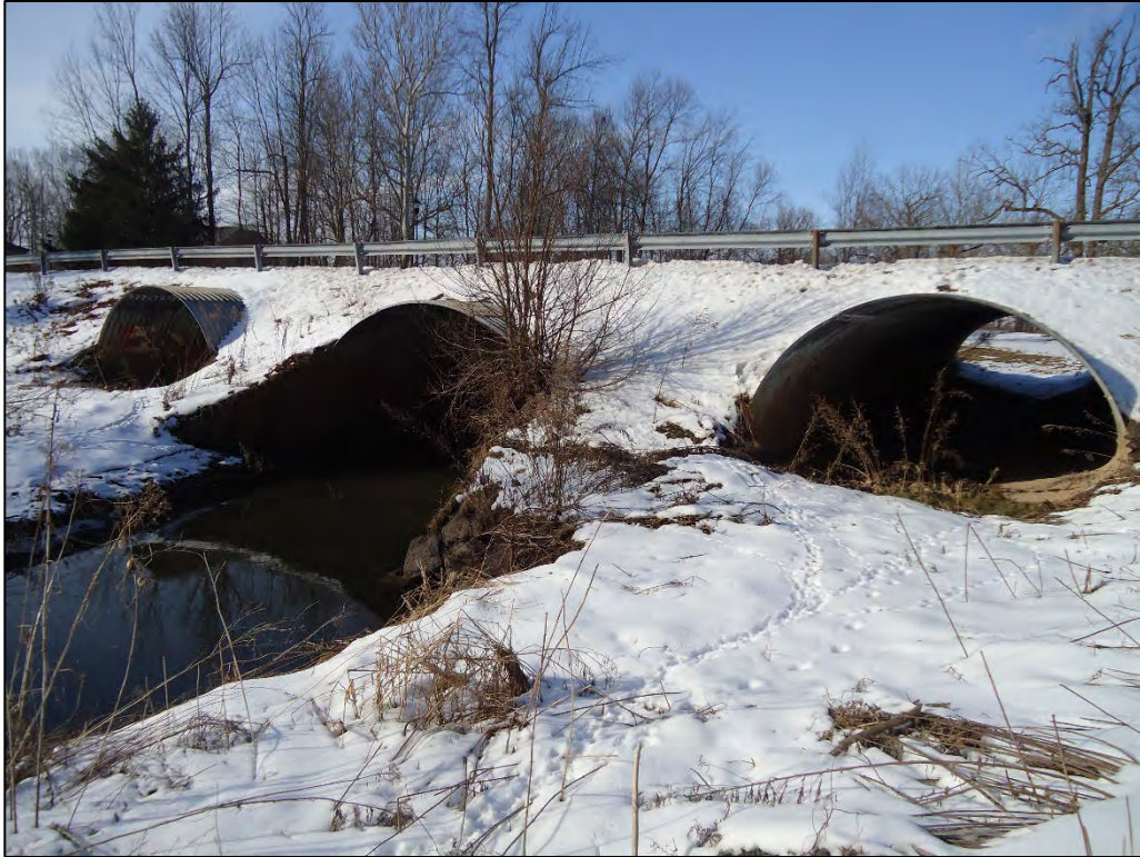
Photo D-6. Upstream face of Glen Oaks Drive culverts for Ransom Creek (2/17/2020)
