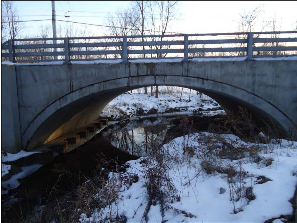
Photo D-10. Downstream face of Miles Road bridge crossing at Ransom Creek (2/17/2020)
