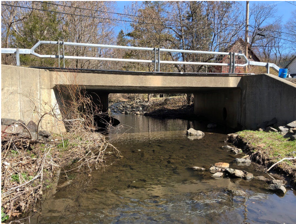
Figure 4-9: Looking upstream through the crossing of Hillside Avenue over the East Branch Saddle River
