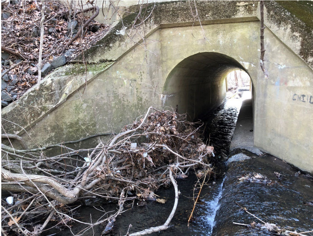
Figure 4-35: Looking at woody debris partially obstructing Conrail structure inlet
