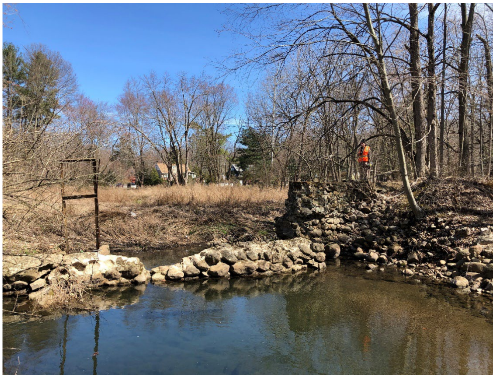
Figure 4-11: Looking upstream at the breached section of the unregistered dam over the East Branch Saddle River at STA 4+50
