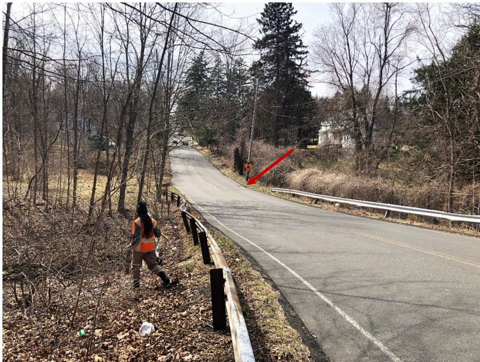
Figure 4-24: Low spot in Christmas Hill Road where culvert gets flanked
