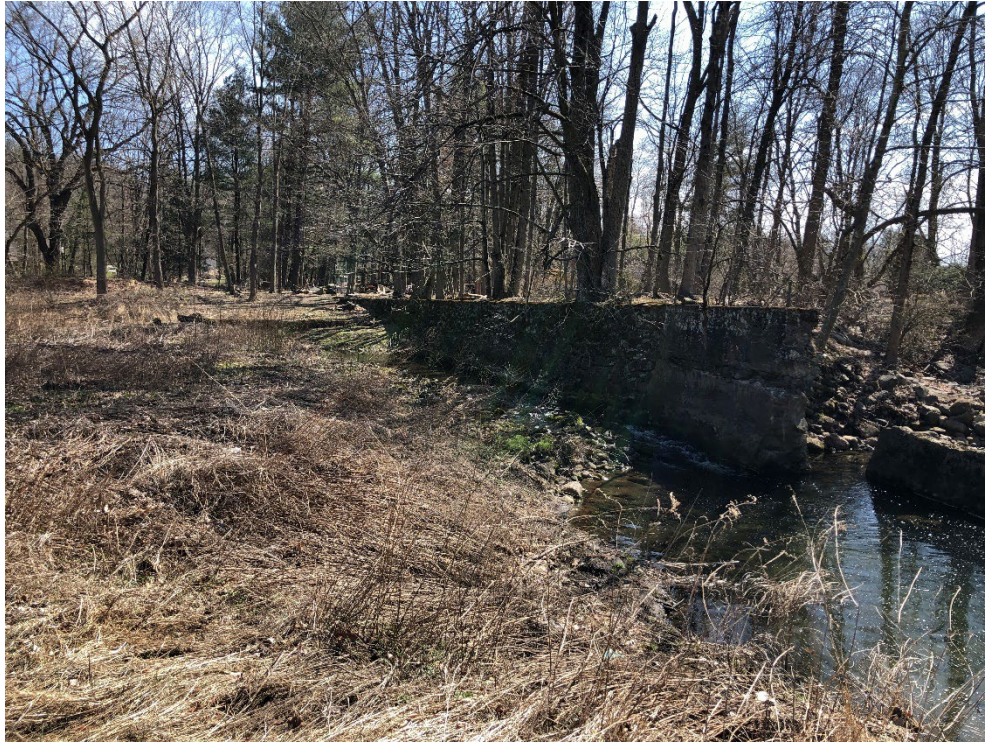
Figure 4-12: Looking downstream at the dam remnants to the left of the breach
