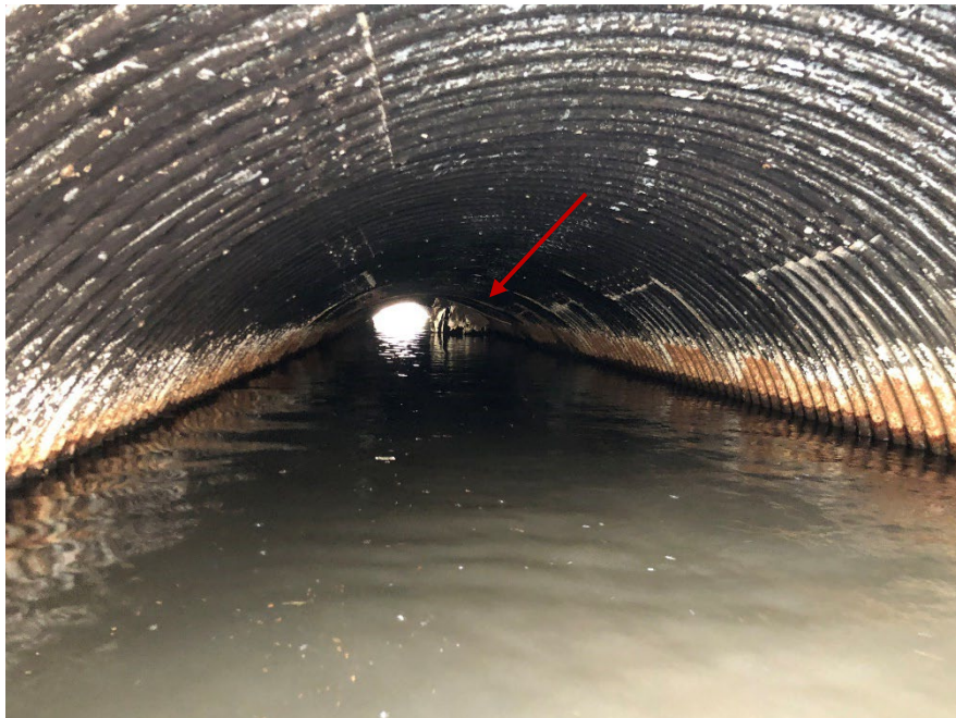
Figure 4-30: Looking downstream at the inside of the river-right culvert. The collapse in the center of the culvert is indicated by the red arrow.
