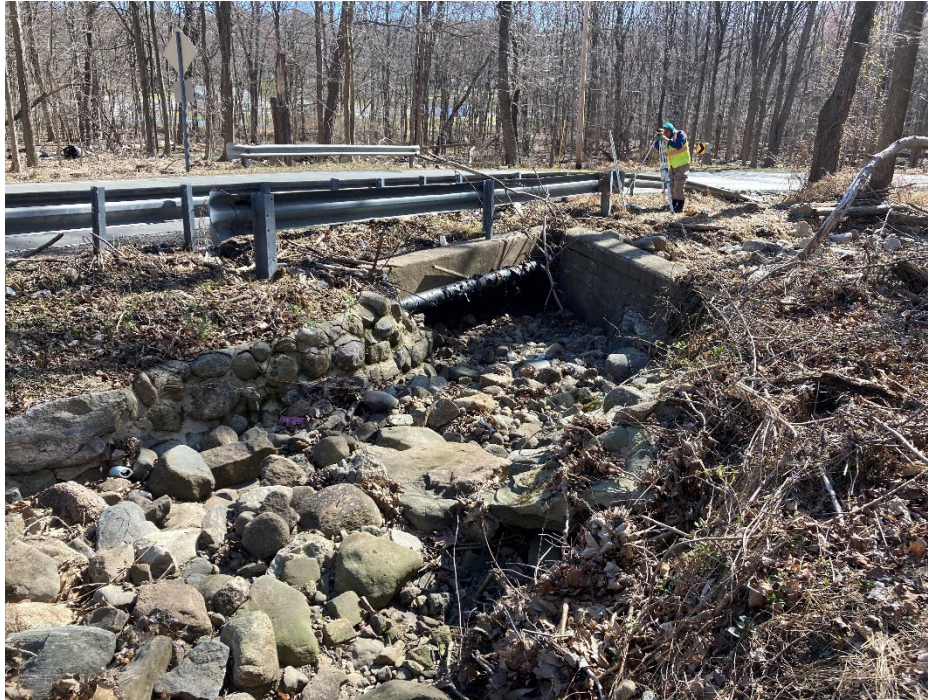
Figure 4-16: Inlet of unnamed tributary of East Branch Saddle River crossing under South Monsey Road
