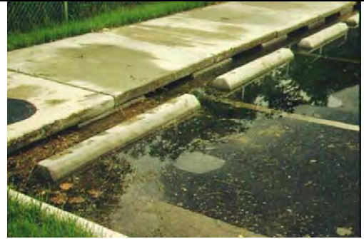
Standing water on the parking lot is evidence that this perimeter sand filter (under the sidewalk) is clogged.
