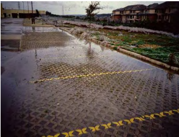
Figure 3.9.1. Winter salting, sanding, plowing, and snow storage can cause problems for permeable pavement surfaces, which will trigger a Level 3 investigation.
