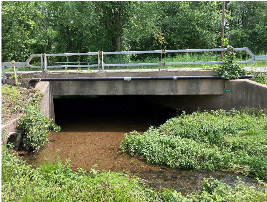
Figure 4-58: Looking Upstream at Route 303 Bridge Outlet Near the Intersection with Mountain View Avenue
