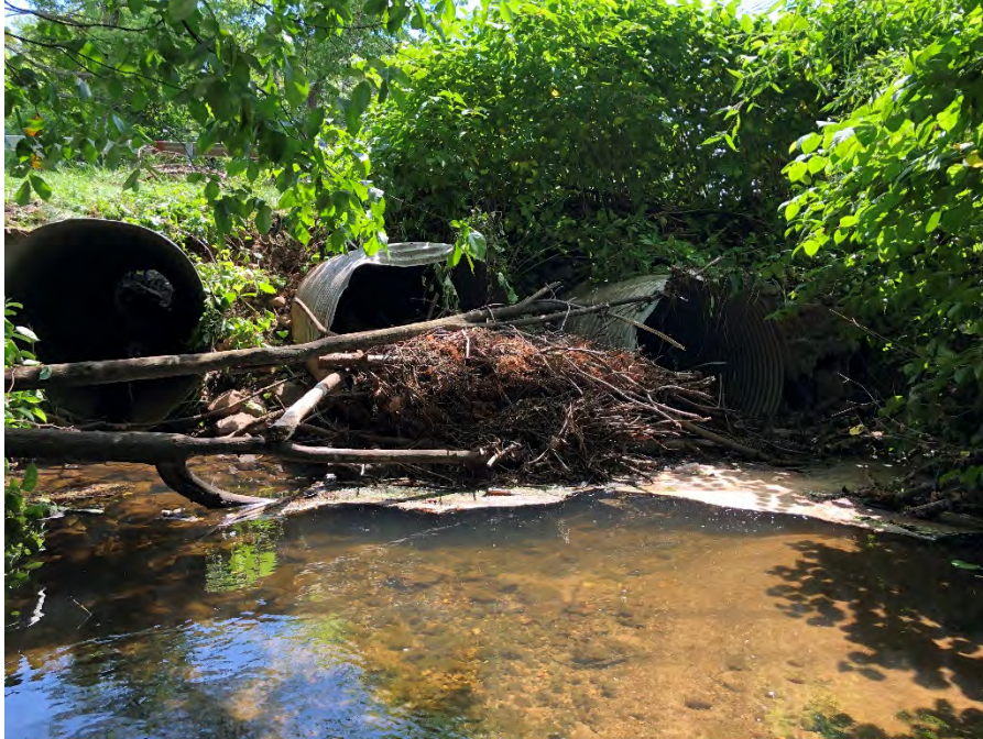
Figure 4-73: Looking Downstream at the Route 340 Culverts, Large Woody Debris Accumulated at the Culvert Inlet
