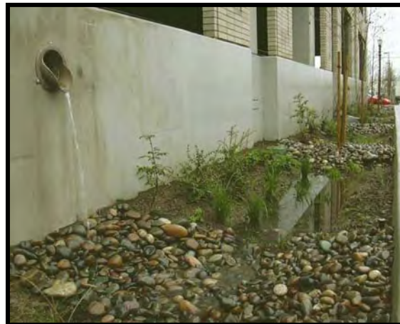
Figure 5: This flow-through planter collects runoff from a parking garage and is incorporated into the structure
