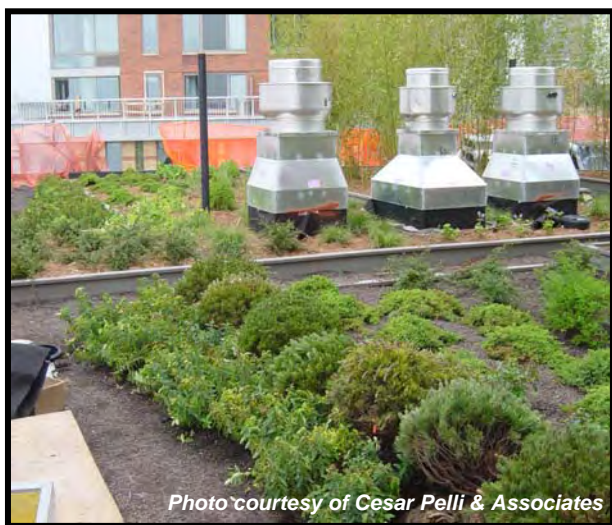
Figure 3: A green roof installed on an apartment building in Manhattan along the Hudson River.
