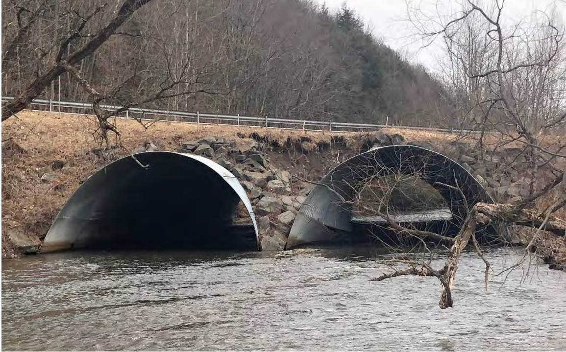
Photo 4-7: Damaged culvert carrying Dug Road over Cold Spring Creek at its confluence with WBDR. View looking upstream. Corrugated arch panels in east barrel have separated, and cover fill is eroding into the creek. Also note sediment aggradation in intermediate slack water.
