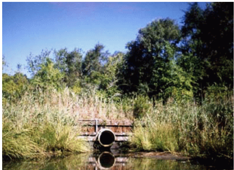
Figure 7. Perched culvert impeding tidal flow.
