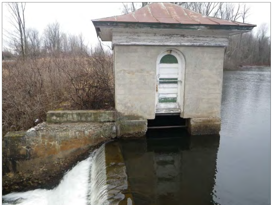
West Pond spillway in deteriorated condition.
