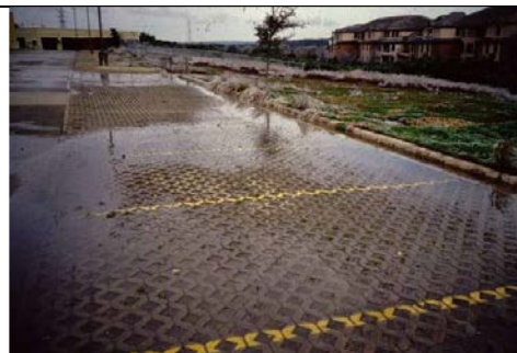
Water standing on the parking surface 48 to 72 hours after a storm is an indication of clogging. Snow piles at the edge of the photo point to possible clogging from winter sanding or plowing.
