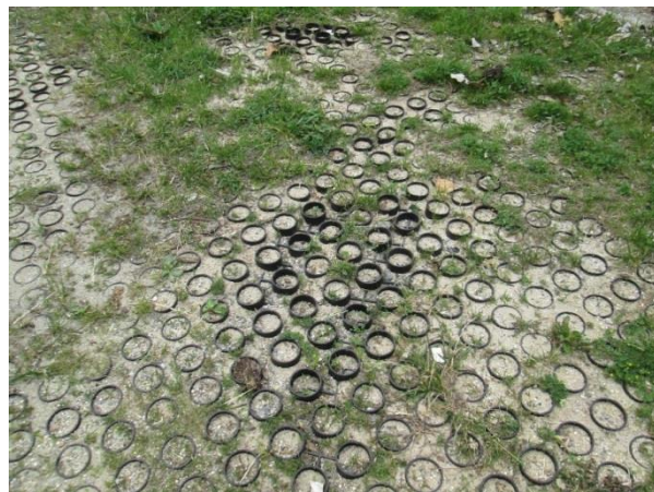
Figure 12.14 A Level 3 Inspection is warranted if more than 25% of the porous pavement surface appears to be clogged, joints are filled in, or vegetation is not growing (as shown in photo).
