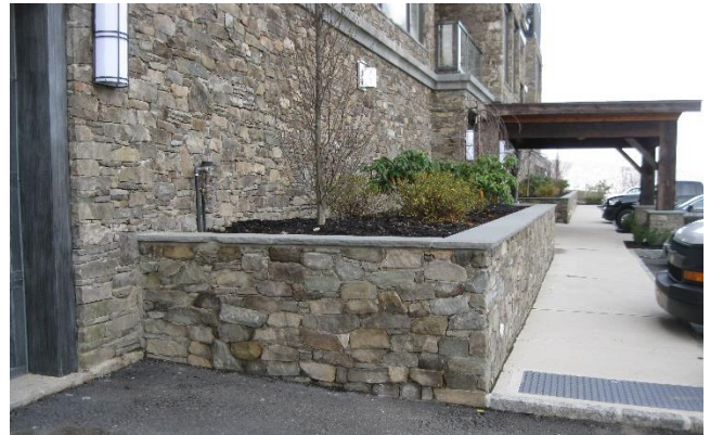
Figure 8.8 Stormwater Planter installed in Tarrytown, NY
