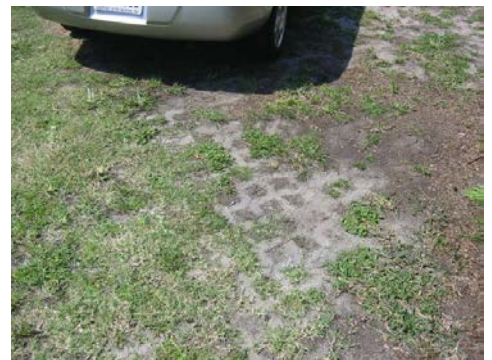
Pulling grass and weeds from the joints can damage parking surface if roots are firmly established in the bedding layer.
