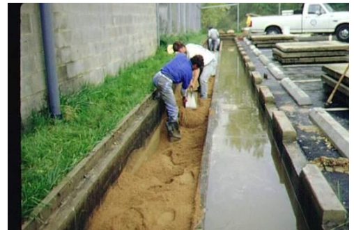
Routine cleaning of a perimeter or "Delaware" sand filter. This can be done from the surface, but deeper, vault-type filters will require confined-space entry procedures.
