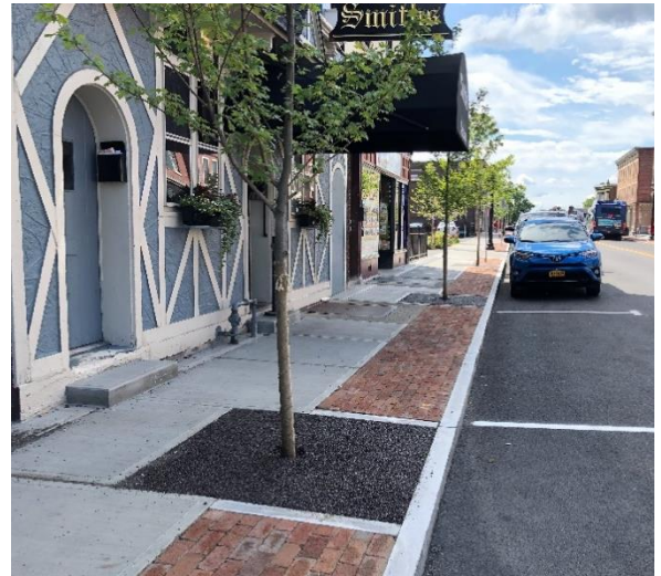
Figure 8.2 Tree Pit installed in Cohoes, NY
