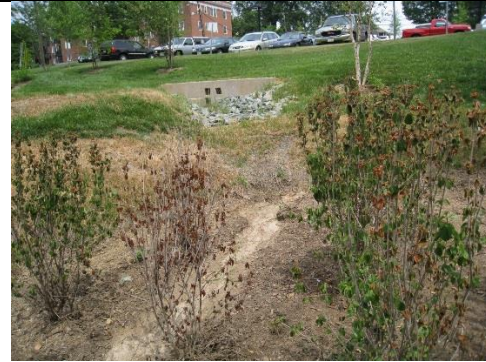
Water from the inlet at top of photo is channeling through the bioretention area.
