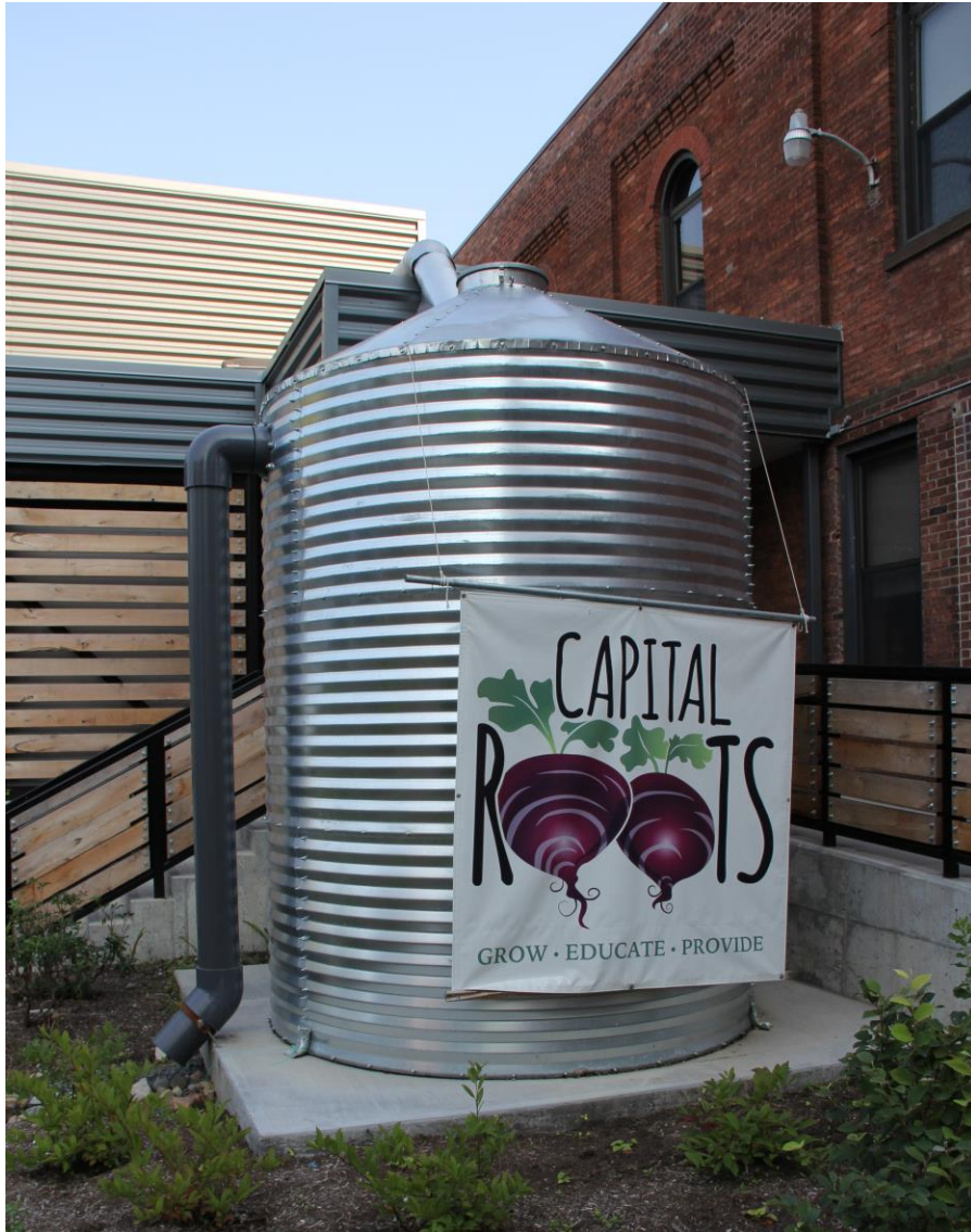
Figure 5.44 Rainwater Harvesting System (RR-8)
