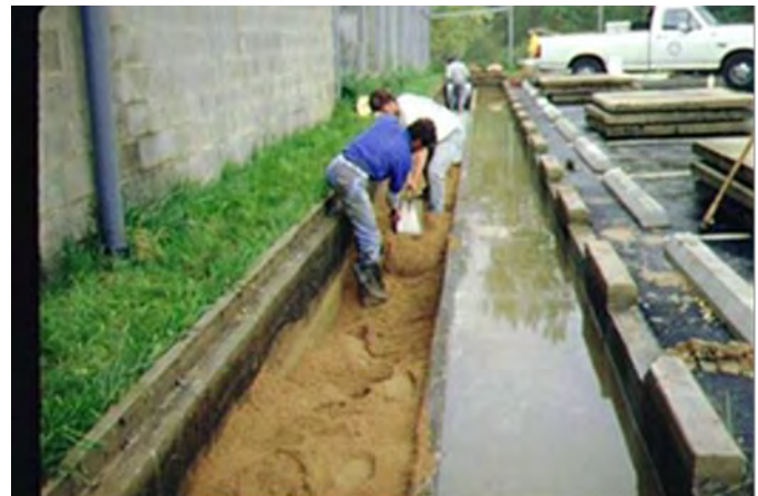
Figure 12.20 Example Concrete Perimeter Sand Filter (photo shows the filter with the grate top off as the filter is being maintained. Sedimentation chamber filled with water is on the right, and the sand filter chamber is on the left.)
