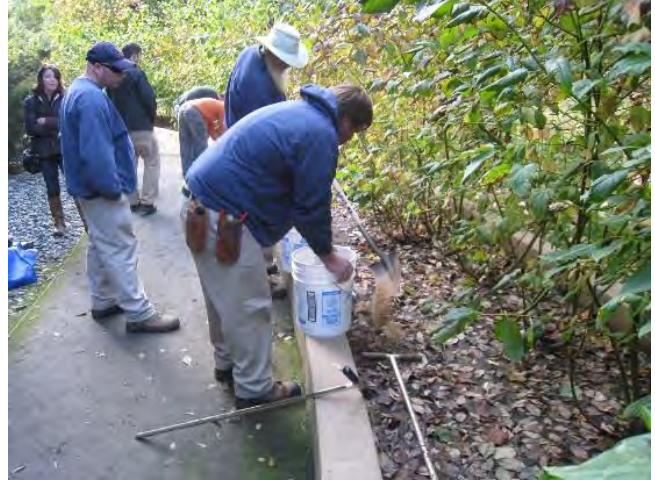
Adding sand to a wick drain. The vertical perforated PVC pipe has already been placed in the auger hole.
