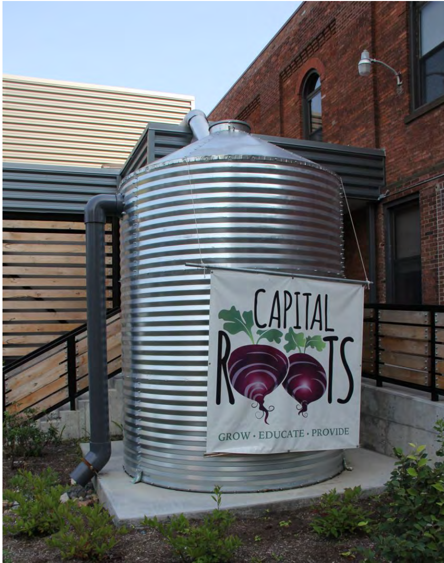
Figure 5.44 Rainwater Harvesting System (RR-8)
