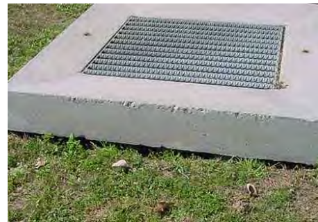
Water is “piping” down to the underdrain at the weak spot where the filter media meets the concrete overflow structure.
