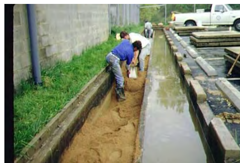
Routine cleaning of a perimeter or "Delaware" sand filter. This can be done from the surface, but deeper, vault-type filters will require confined-space entry procedures.
