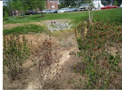
Water from the inlet at top of photo is channeling through the bioretention area.
