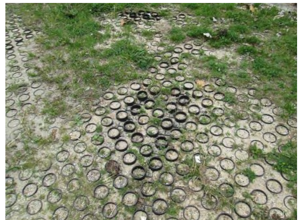
Figure 12.14 A Level 3 Inspection is warranted if more than 25% of the porous pavement surface appears to be clogged, joints are filled in, or vegetation is not growing (as shown in photo).
