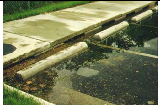
Standing water on the parking lot is evidence that this perimeter sand filter (under the sidewalk) is clogged.
