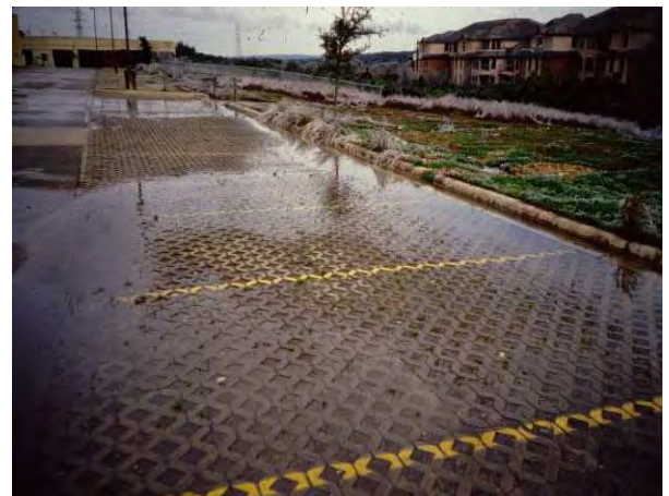
Figure 12.13 Winter salting, sanding, plowing, and snow storage can cause problems for porous pavement surfaces, which may trigger a Level 3 Inspection.
