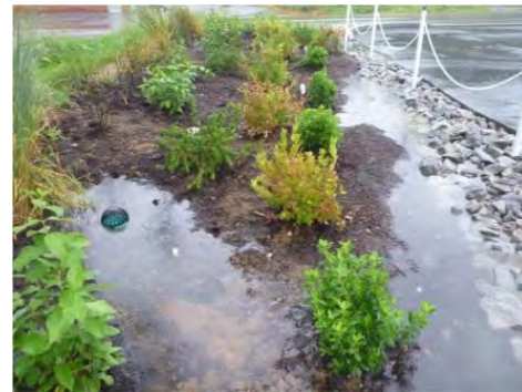
Water is preferentially ponding only at one end of the bioretention because the surface is not flat.
