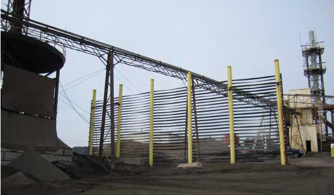
Figure 1. Wind Screen in Finish Plant Area
