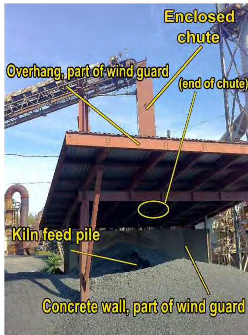
Photo 6. Kiln feed pile, showing concrete wind wall in back, metal overhang, and chute above pile.
