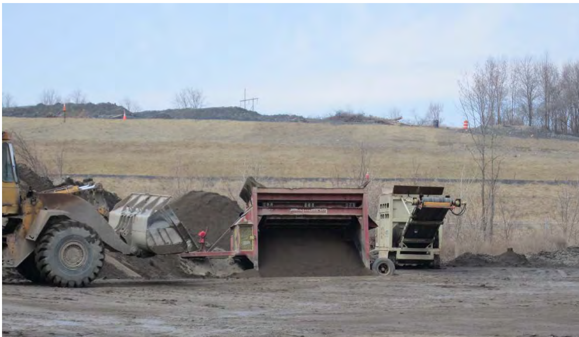
Figure 9. Portable Screens in the Block Mix Processing Area
