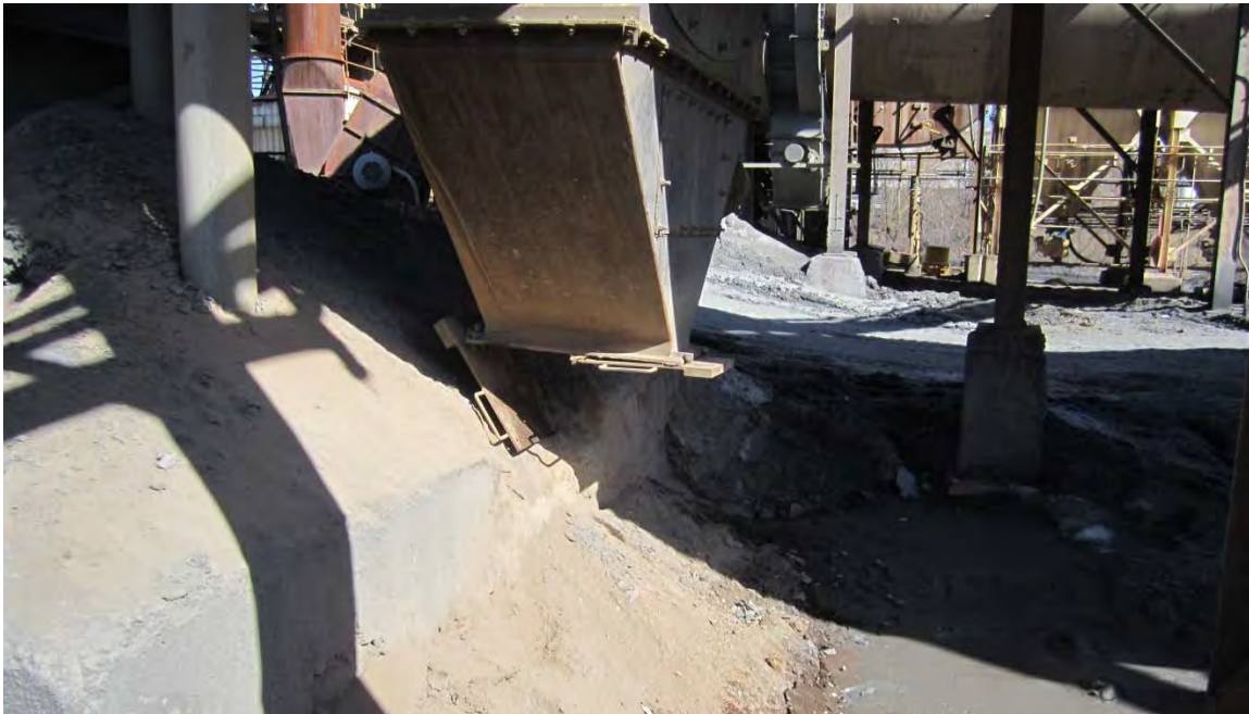
Figure 5. Chute for Cleaning Kiln Rim Seal
